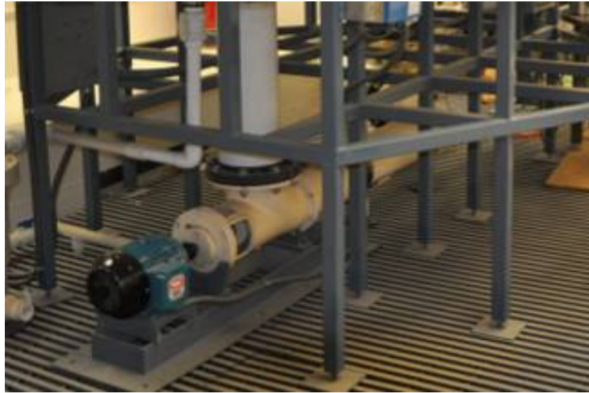
Figure 12. Water Tunnel Two pump.
