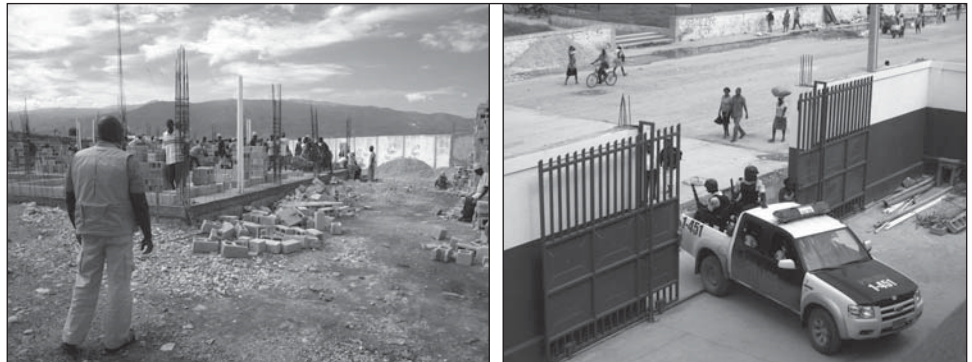
Figure 8: Construction and Renovation of Police Buildings under Section 1207 Program to Help Stabilize the Cité Soleil Neighborhood in Port-au-Prince, Haiti, September 2009
