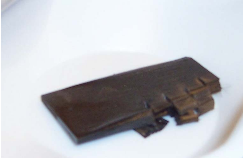
Figure 7 Burnt ticket post cut with obvious flaking off of material due to delamination
