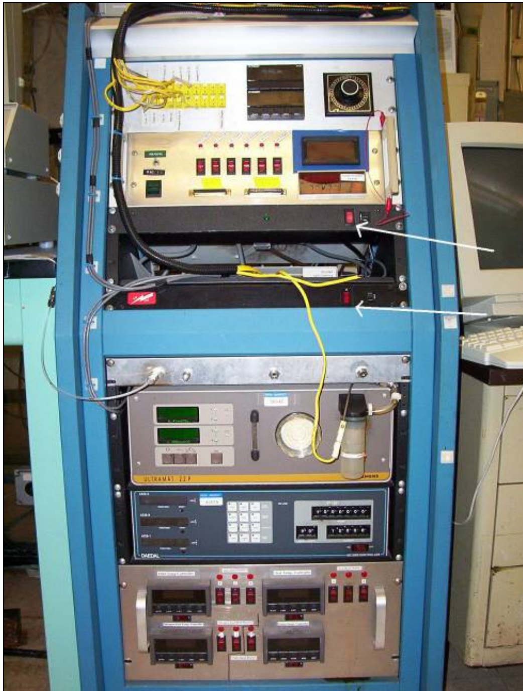
Figure A.1: Picture of PFR controllers with arrows identifying main power supply control switches.
