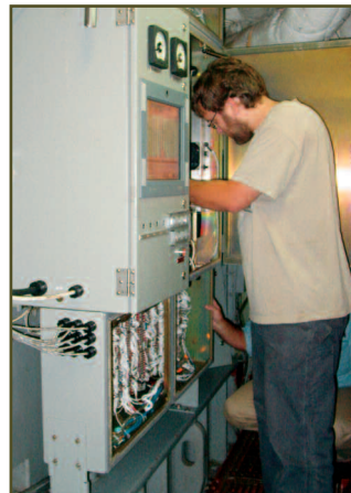
Left: Carderock Division engineers Jeremy Nichols (standing) and Brian Connery troubleshoot the No. 2 Gas Turbine Generator (GTG) Full Authority Digital Control (FADC) Load Control Panel (LOCOP) aboard USS Vella Gulf (CG 72).
