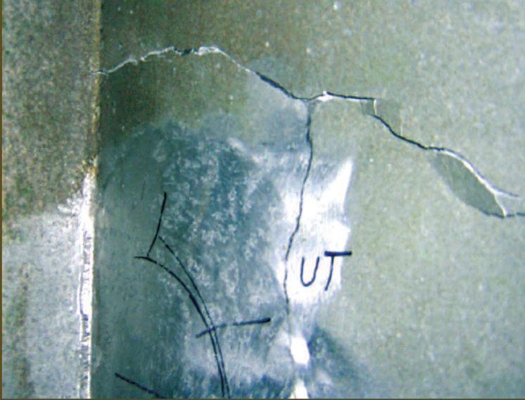
Above: Stress corrosion cracking in a non-structural bulkhead of a Ticonderoga Class cruiser.
