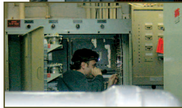
Above: Carderock Division engineer Chris Corso conducts the Generator Control Unit (GCU) checkout procedure aboard USS Princeton (CG 59).
