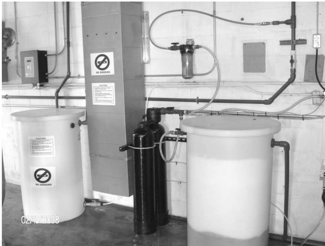
Figure 3. In-line components of the MIOX biocide-generating system.
