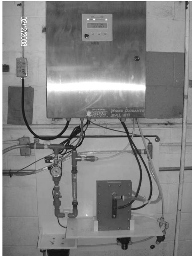
Figure 2. MIOX control panel (top) and electrolytic cell (bottom).
