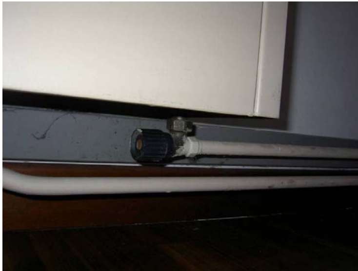
Figure 26. Manual radiator valve.
