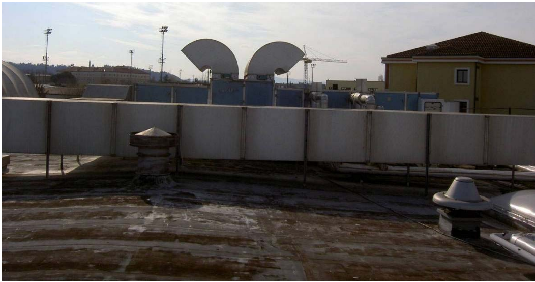
Figure 16. Roof top air handling units at Bldg 311.
