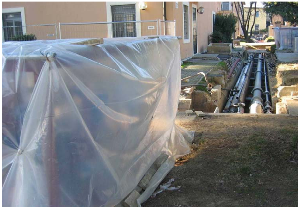
Figure 13. New Heat exchanger stations.
