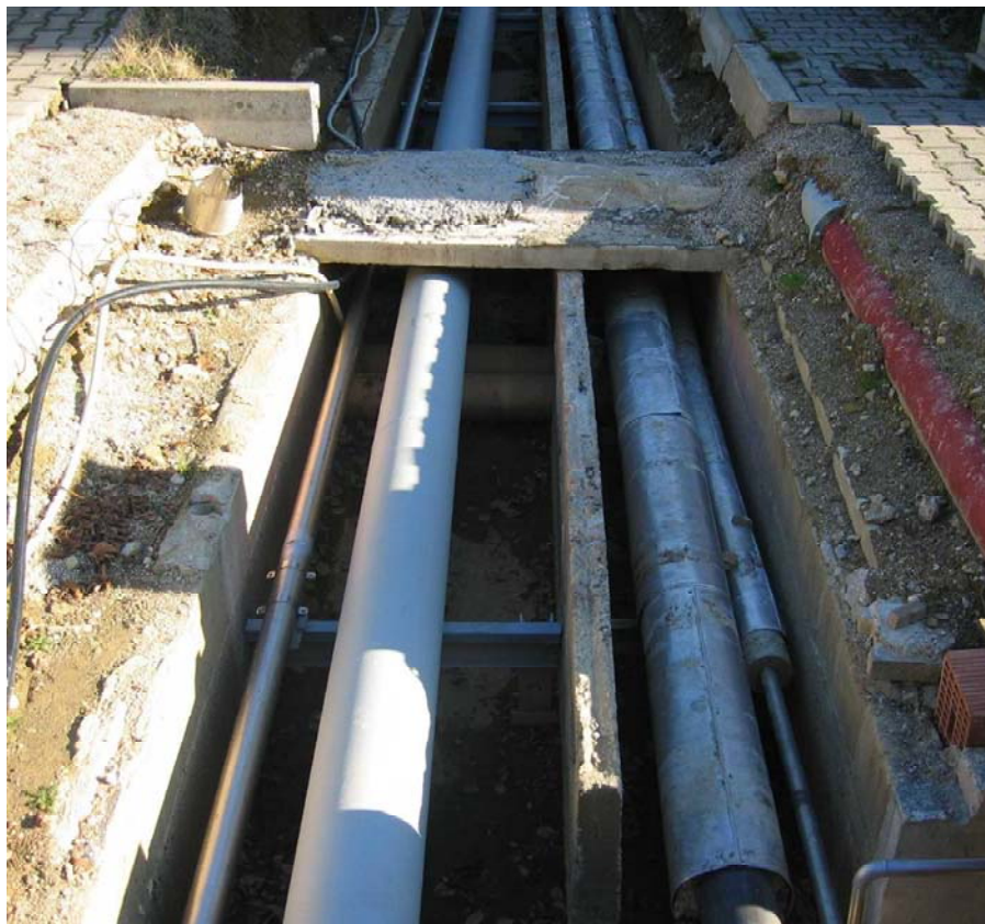
Figure 12. New steam and condensate lines.
