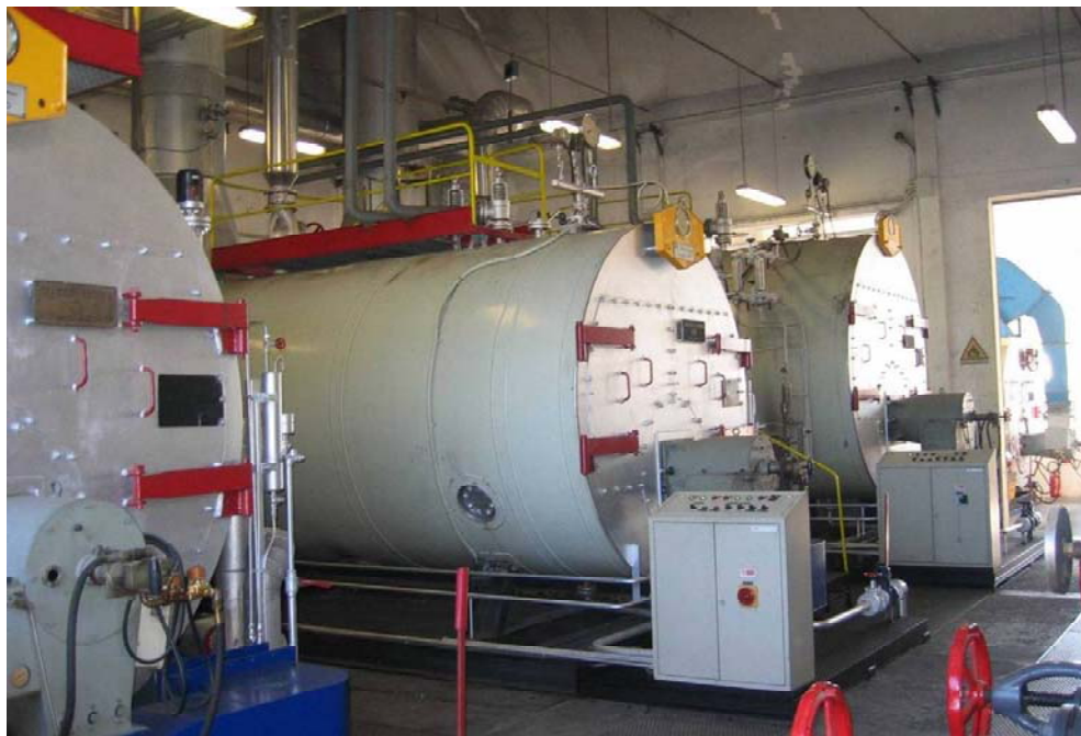
Figure 10. Steam Boilers in Bldg 206.
