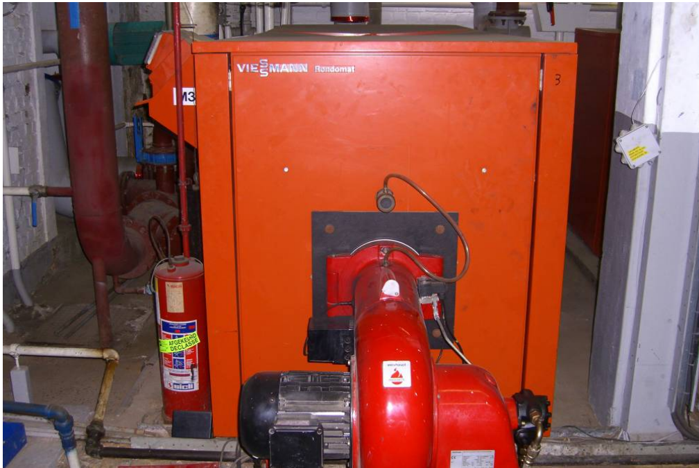
Figure 9. One of the three boilers of the district heating plant.
