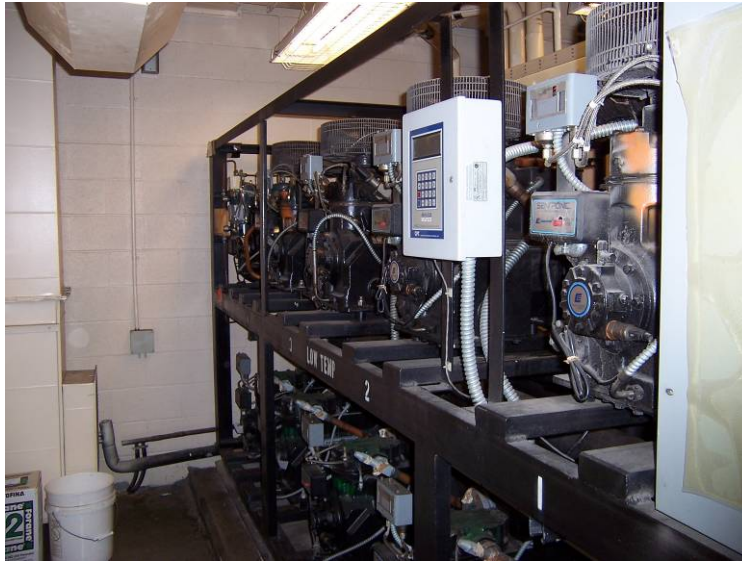
Figure 26. Rack of refrigerated room compressors.
