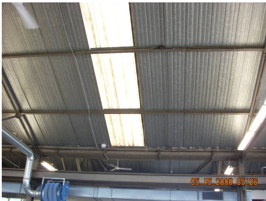
Figure 31. Picture of skylights in Bldg 34 showing dirty skylights and lights on.
