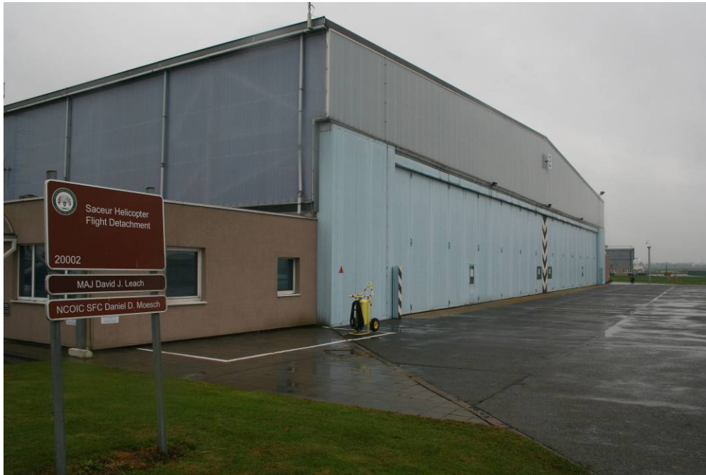
Figure 7. Door on one side of Bldg 2002 that has opening under rail.
