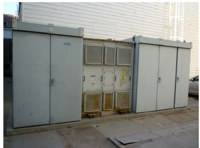
Inefficient HVAC System at Naval Base San Diego, CA
