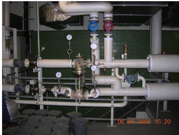
Figure 41. Substation of Bldg 4a (hangar).
