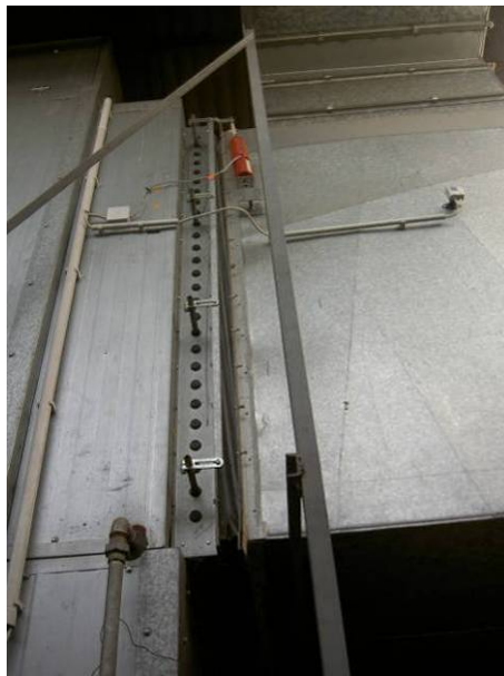
Figure 29. Bldg 18 OA damper.
