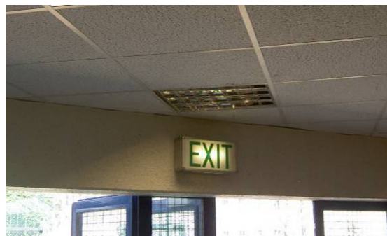
Figure 32. Fluorescent light exit sign.
