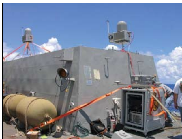
FIGURE 7 TEWM installed on the DDG 93 Chung Hoon .
