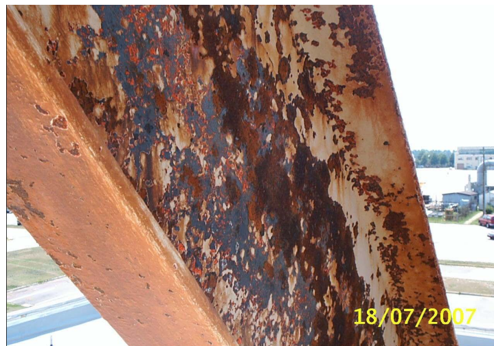
Figure 28. Condition of hangar superstructure before work began.
