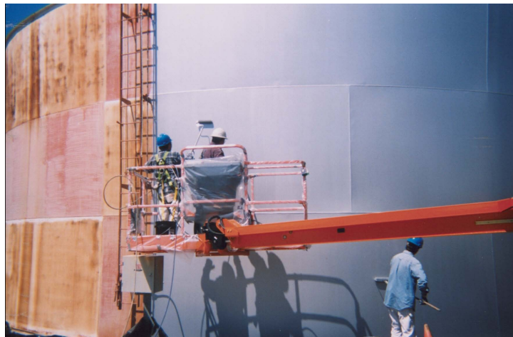
Figure 34. Priming a deluge tank.
