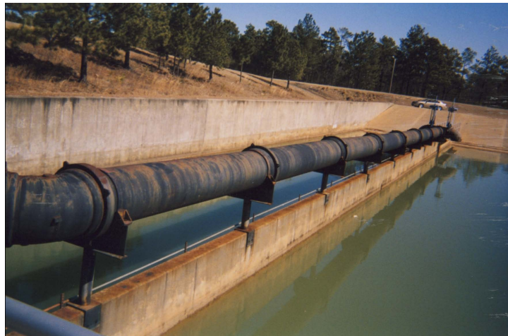
Figure 24. Pipe before abrasive blasting showing corrosion.
