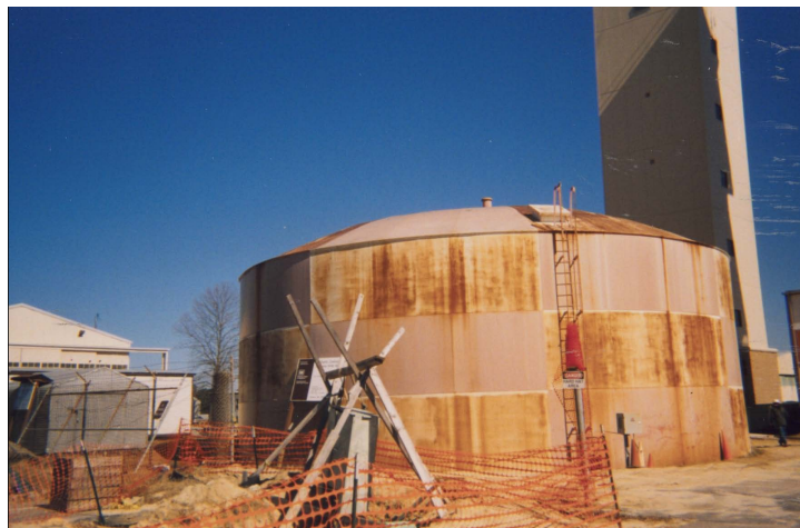
Figure 2. Deluge Tank No. 2 before painting.
