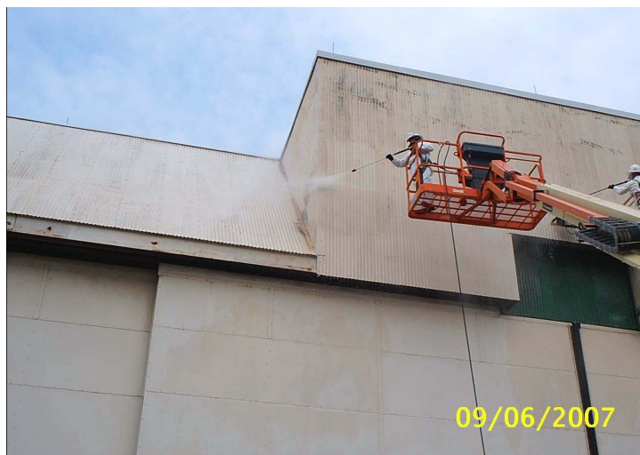
Figure 14. Simmons AAF hangar during power washing to remove dirt, chalk, and loose paint.
