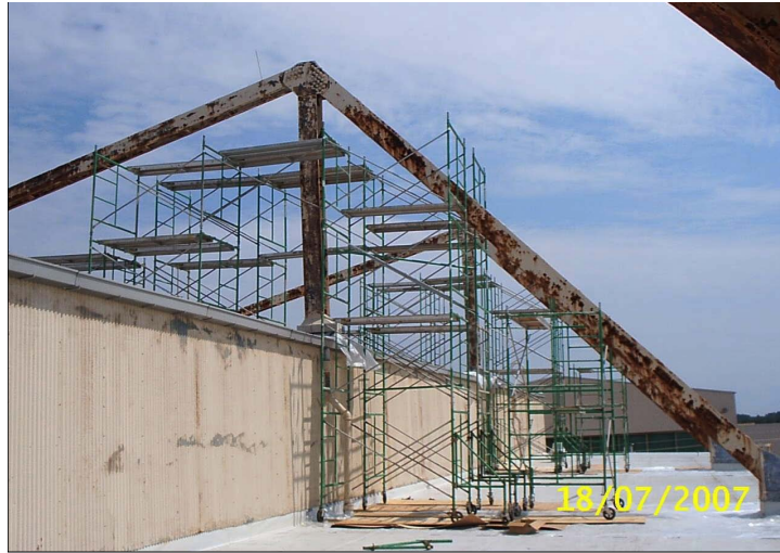
Figure 15. Simmons AAF hangar before overcoating. Note the extent of rust on the steel superstructure and metal siding.
