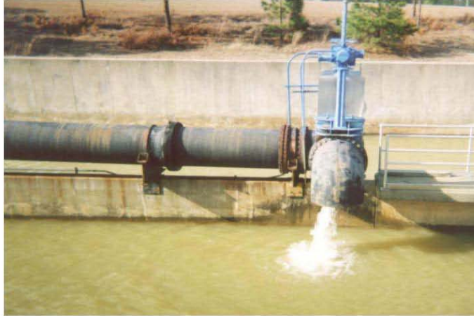
Fig. 2. Close-up of Inlet Pipe (2 ft. diameter) at Ft. Bragg Central Vehicle Wash Facility (CVWF) showing severe coating degradation
