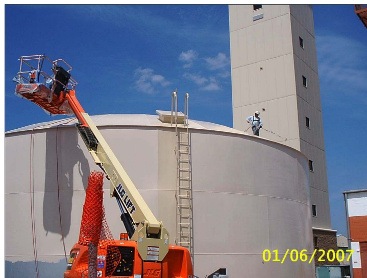
Figure 37. Applying topcoat to tank roof using a power roller. All work was performed by brush and roll to prevent overspray damage to vehicles and facilities.
