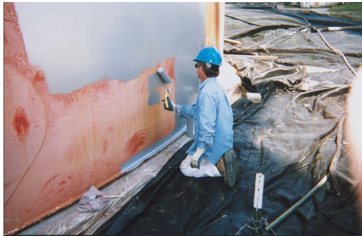
Figure 33. Priming a deluge tank.
