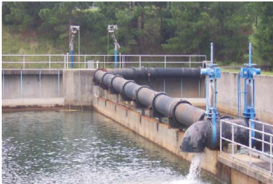
Figure G1. CVWF inlet pipe, May 2007.
