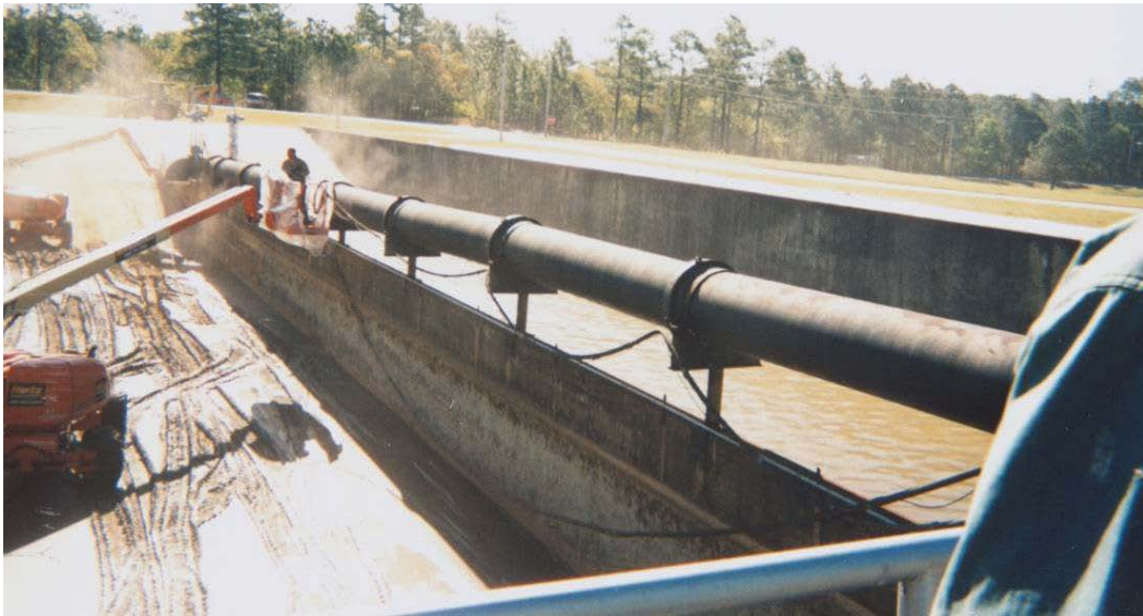
Figure 9. Surface preparation of the inlet pipe of CVWF grit settling chamber prior to coating with smart coatings.
