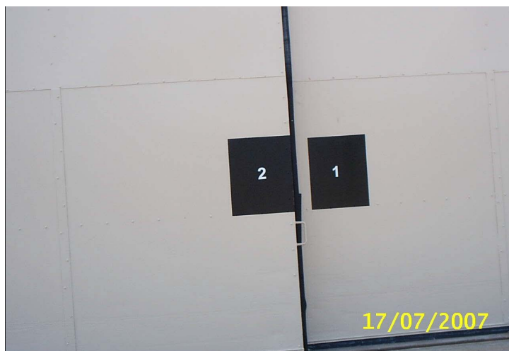
Figure 8. Simmons AAF hangar doors after overcoating.
