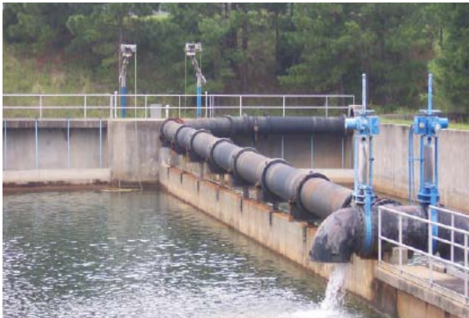
Figure 2. Corroded inlet pipe at the CVWF grit settling chamber.
