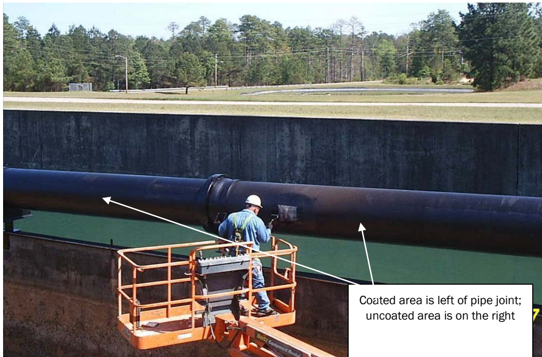
Figure 11. Inlet pipe of CVWF grit settling chamber being coated with coal tar epoxy that with self healing and fluorescent additives.
