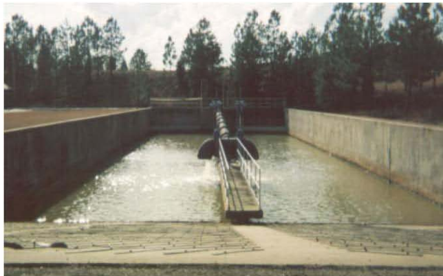
Fig. 1. Fort Bragg Central Vehicle Wash Facility (CVWF) Grit Settling Chamber showing inlet pipe.
