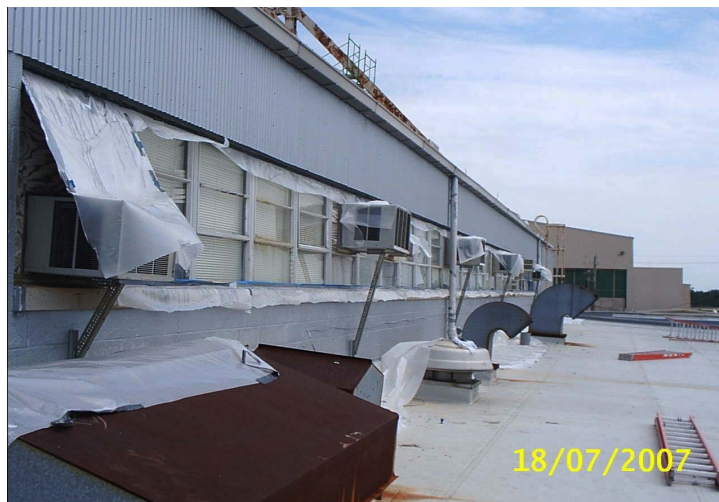
Figure 11. Simmons AAF hangar after first MCU coat, showing protective covers and masking.
