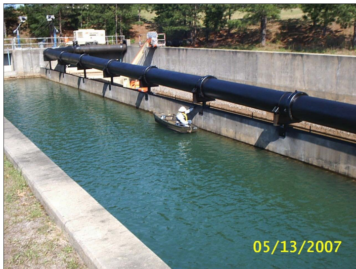
Figure 19. Smart coatings on pipe at CVWF grit basin.
