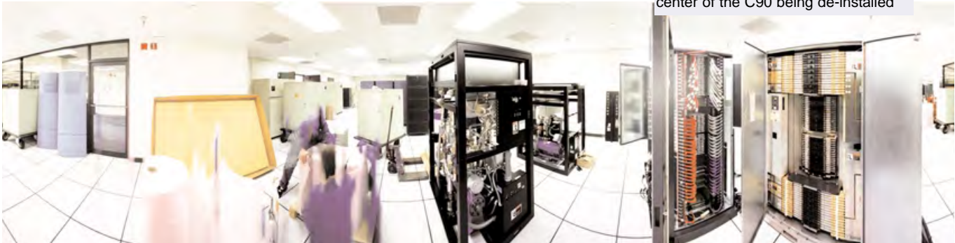
A panoramic view in the operations center of the C90 being de-installed
