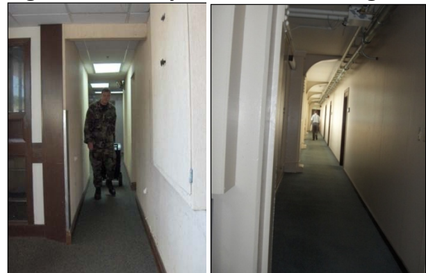
Figure 2. Hallways Too Narrow for Egress
