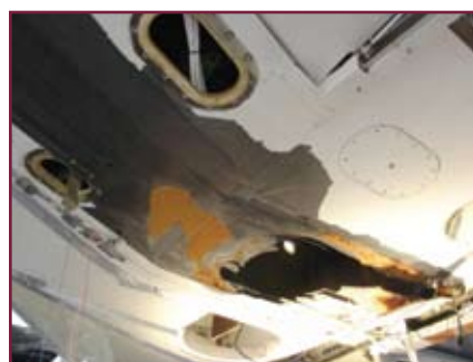
Figure 5 HEI Wet Bay Top Damage
