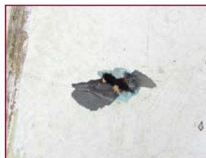
Figure 6 12.7-mm Wet Bay Damage
