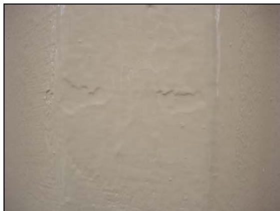
Figure 40: Area after MANTA repaired damage
