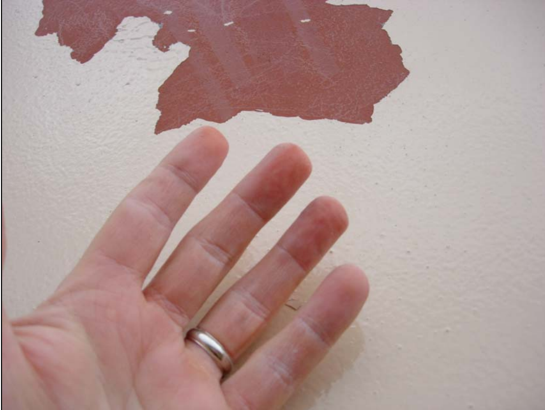
Figure 8: Chalk seen on fingers after rubbing on coated surface where delamination occurred
