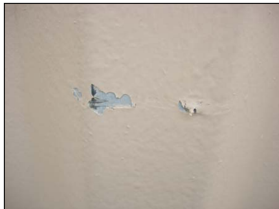
Figure 39: Damage to paint from gate latch
