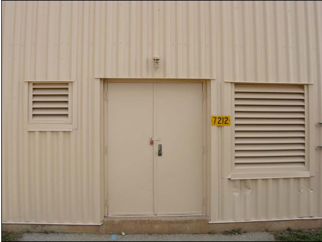
Figure 34: Dented siding on Flight Control Tower beneath the large vent
