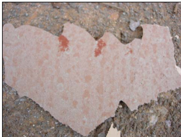
Figure 9: Backside of coating that delaminated
