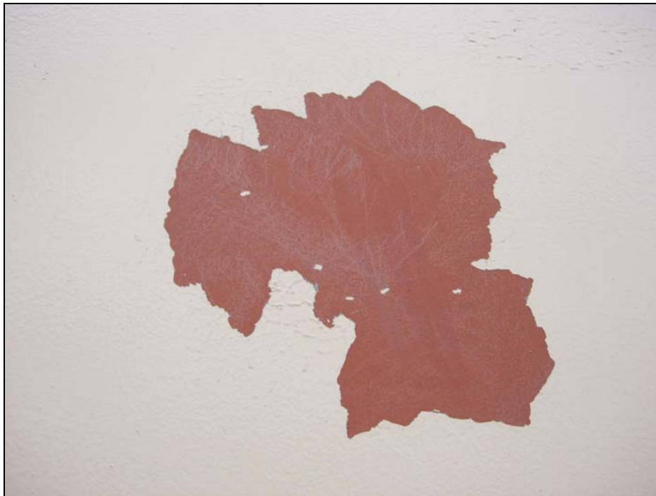
Figure 7: Close up of area shown in Figure 6
