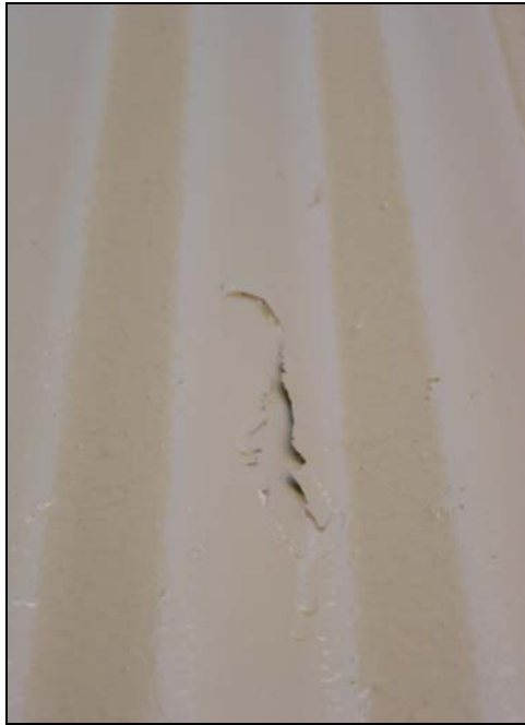
Figure 23: Loosely adhered coating
