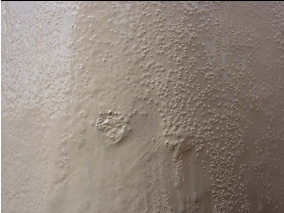
Figure 32: Small bubbles in the Sherwin Williams Corothane I Ironox topcoat
