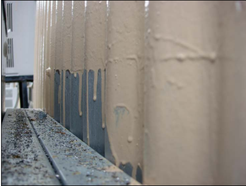
Figure 27: Difficult to access area that was not primed or topcoated
