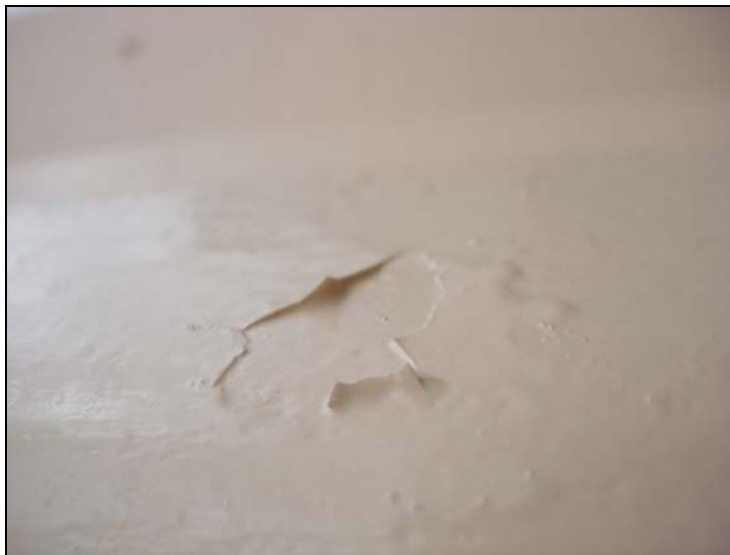
Figure 35: Edges of coating are not adhered to the surface
