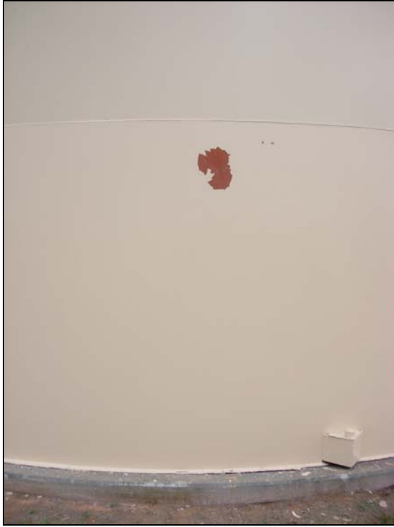
Figure 6: Long view of delaminating paint
