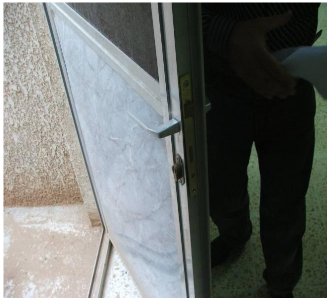
Site Photo 24. Low quality door latch
