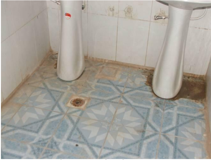
Site Photo 22. Leaking lavatory
