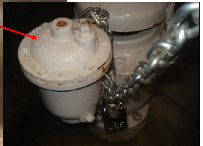
Site Photo 5. Close up of Site Photo 4
