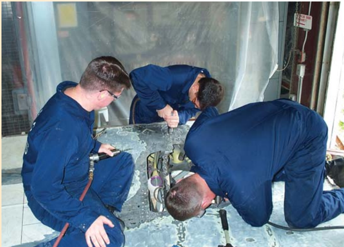
TSgt Tim Fugere (649 th CLSS), TSgt Richard Cousineau, and SSgt Sean Dolney (653 rd CLSS) perform fastener removal on the upper wing structure.
