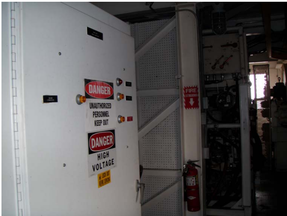
Photograph 80: Interior electrical equipment in the Tether Building.
