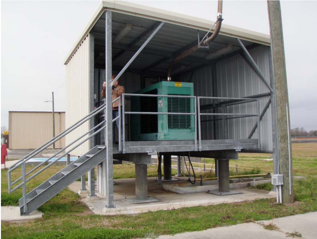
Photograph 63: Generator Enclosure and generator. Yellow aboveground fuel line can be seen underneath the enclosure.
