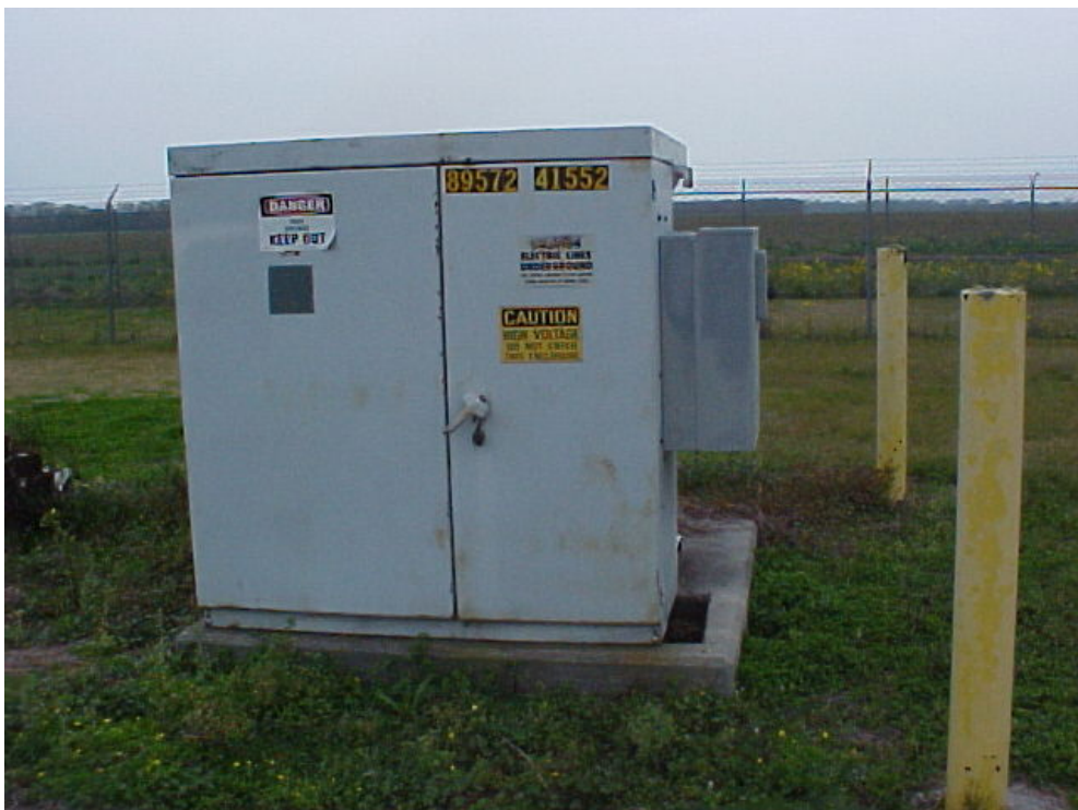
Photograph 84: Closer view of same transformer on southeast section of site.
