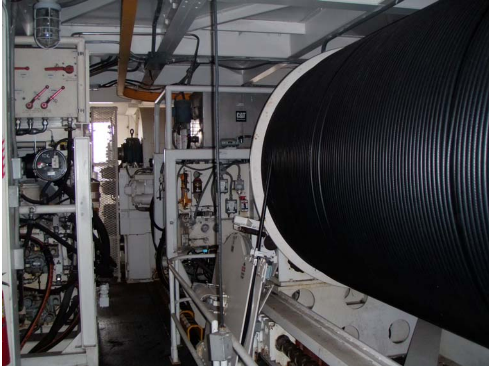
Photograph 81: Mechanical, hydraulic, and tether cable equipment in the Tether Building.
