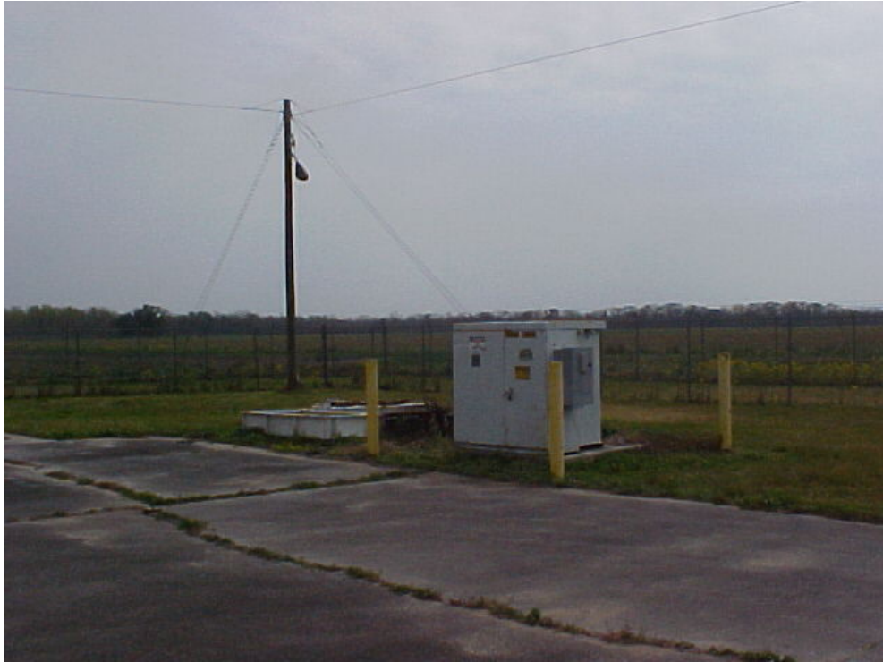
Photograph 83: Site Transformer. Southeast section of site.
