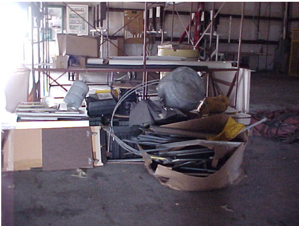
Photograph 53: Rubbish piles in the Payload Service Building #003.
