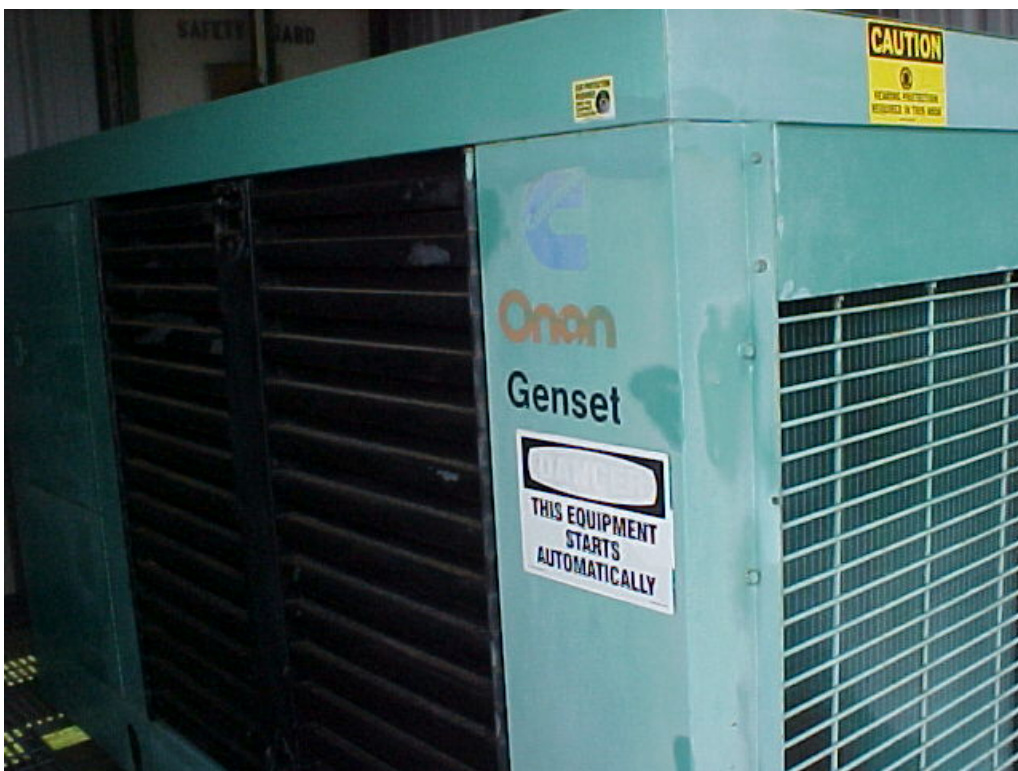
Photograph 64: Generator located in the Generator Enclosure.
