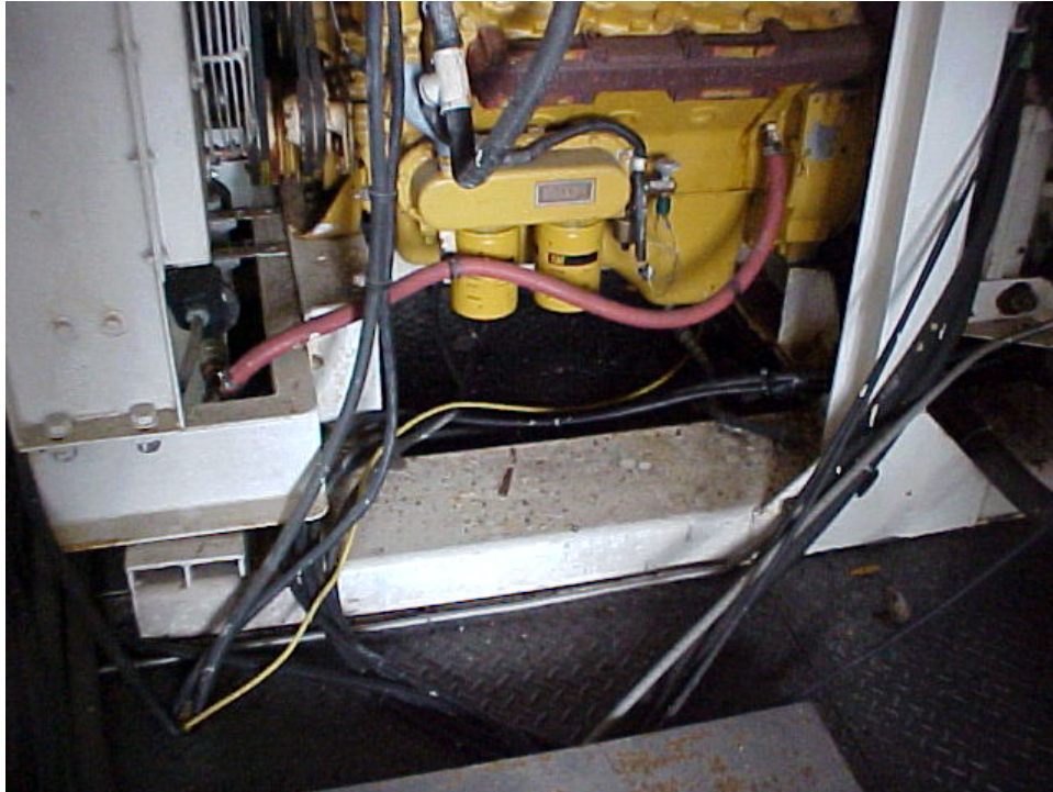
Photograph 79: Interior of the Tether Building. Fluid loss was observed on the floor underneath the motor.
