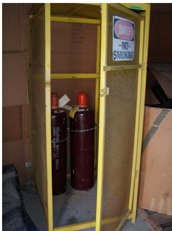
Photograph 54: Acetylene cylinders located in Payload Service Building #003.
