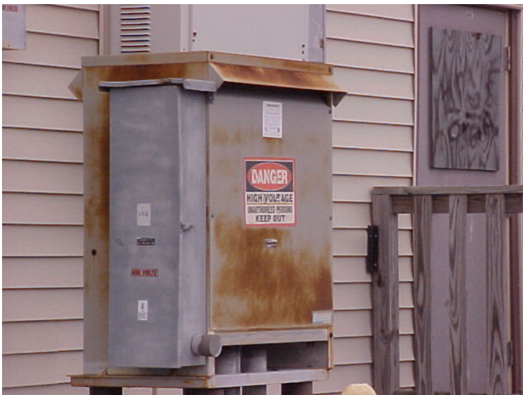
Photograph 8: Transformer outside the Operations Building #001; east wall shown above.
