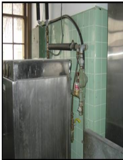
Figure 2. Deteriorated Dining Facilities
