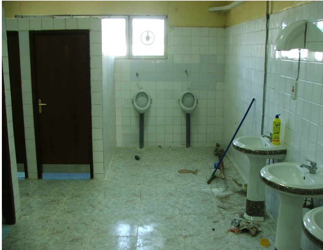
Site Photo 15. Bathroom with Additional Repairs Required
