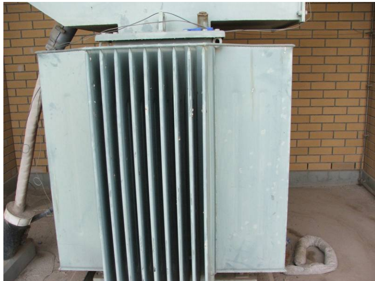
Site Photo 4: Transformer located at S-330
