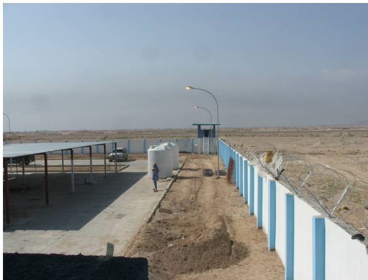
Site Photo 9: 8-meter light poles
