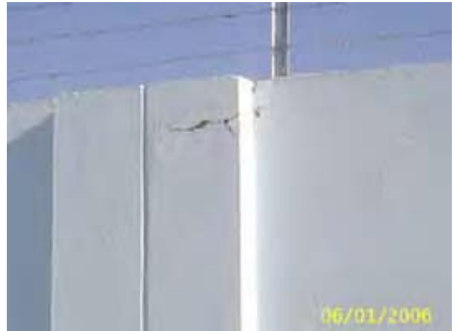
Site Photo 63: Crack in perimeter wall (Project 19111)
