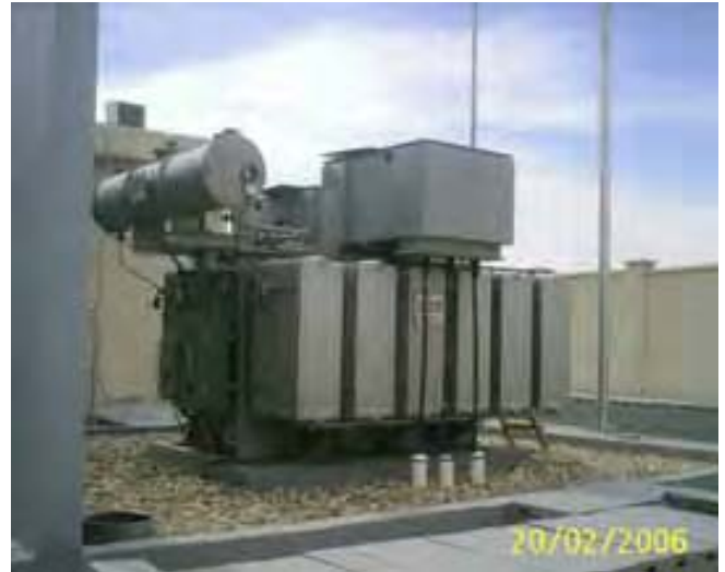
Site Photo 44: Transformer (Project 1861)
