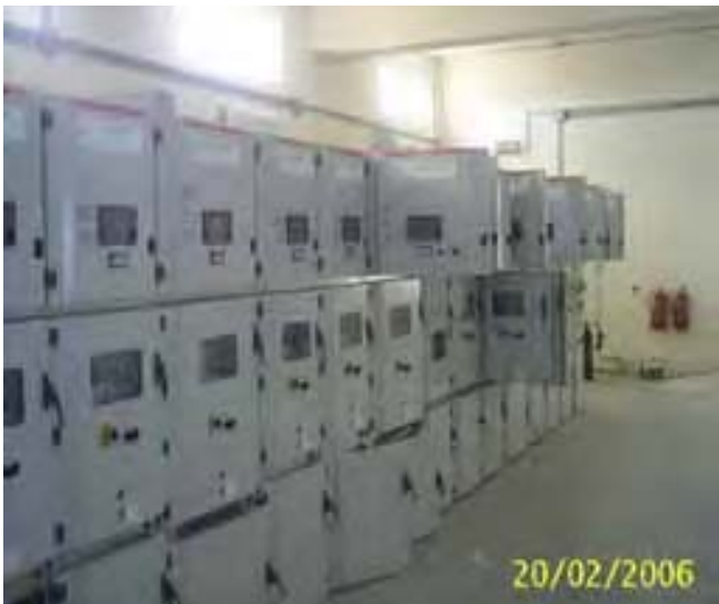
Site Photo 45: Switchgears (Project 1861)
