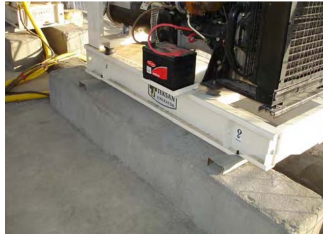
Site Photo 21: Generator on concrete base (Project 12850)
