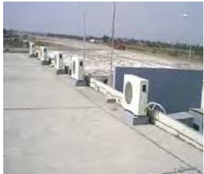
Site Photo 46: Roof mounted AC Units (Project 1861)
