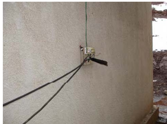
Site Photo 40: Exterior electrical wiring
