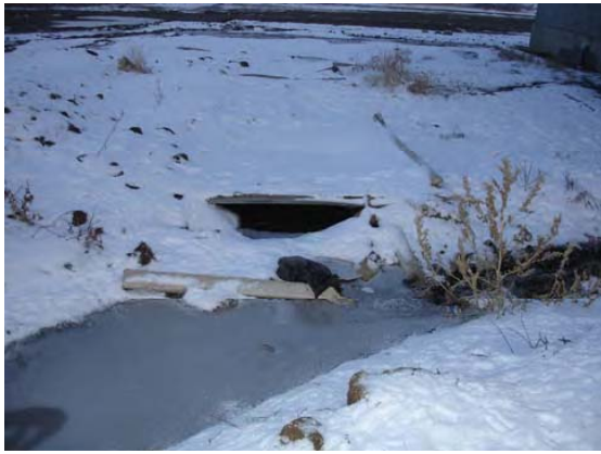
Site Photo 37: Sewage overflow area (Project 20575)
