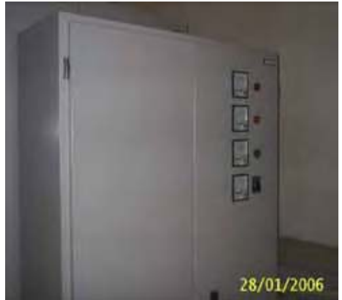
Site Photo 57: Electrical controls (Project 11913)
