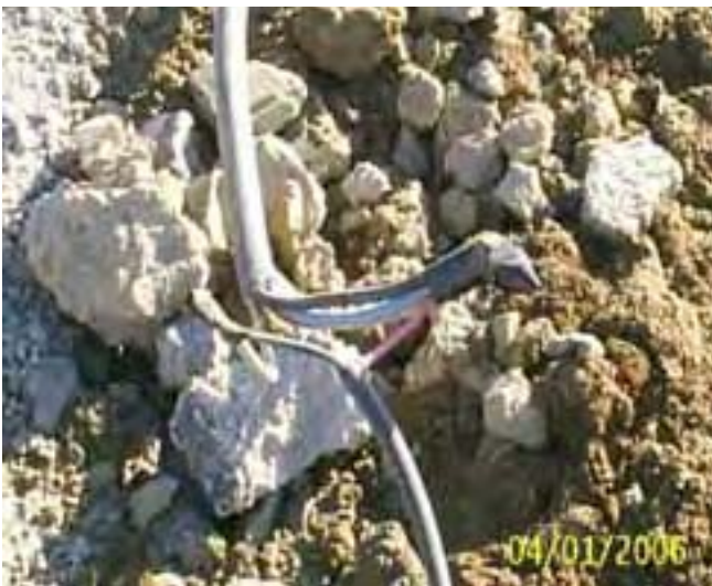
Site Photo 72: Exposed electrical wirings (Project 19179)
