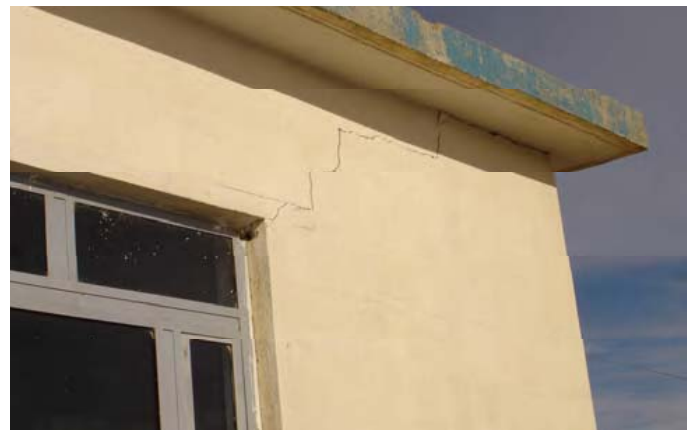
Site Photo 33: Cracks in exterior wall (Project 20572)
