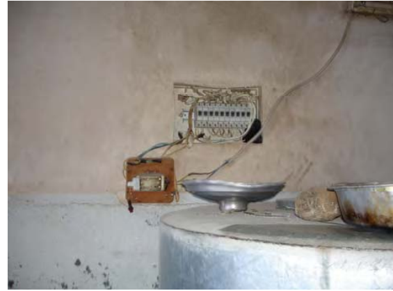
Site Photo 38: Electrical panel (Project 20575)
