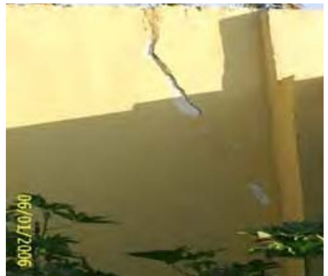
Site Photo 79: Crack in perimeter wall (Project 19227)
