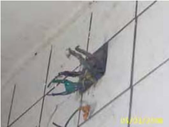
Site Photo 74: Exposed electrical wirings (Project 19181)
