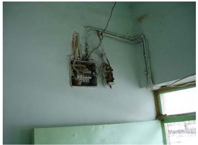
Site Photo 42: Interior electrical panel (Project 20577)
