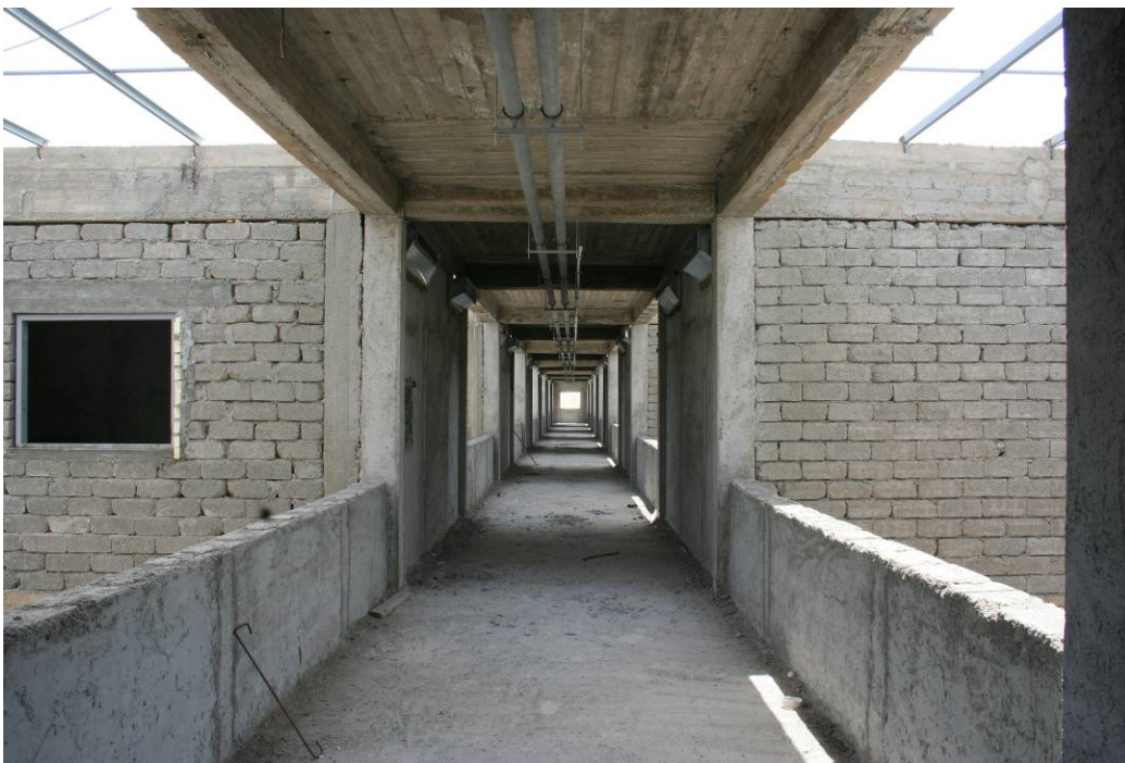
Site Photo 22. Corridor contains firefighting system piping.
