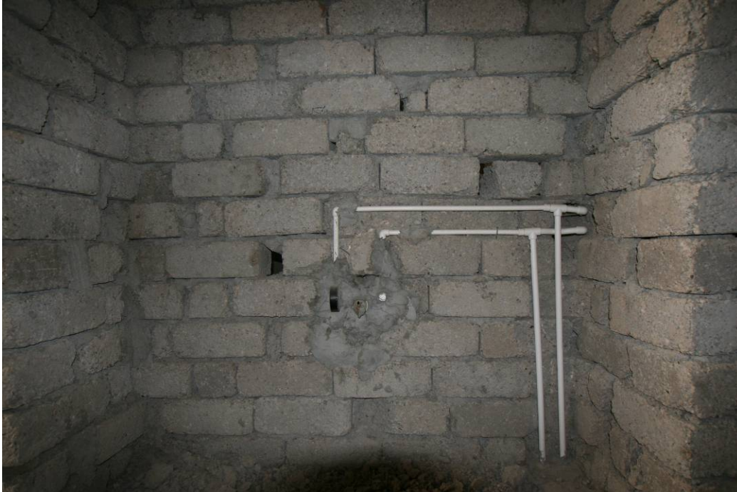
Site Photo 21. Wall installation of bathroom area domestic water pipes before finishing.
