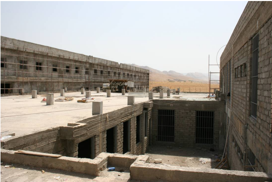
Site Photo 12. Left side of photo shows completed exterior finish work, while right side shows an unfinished wall.
