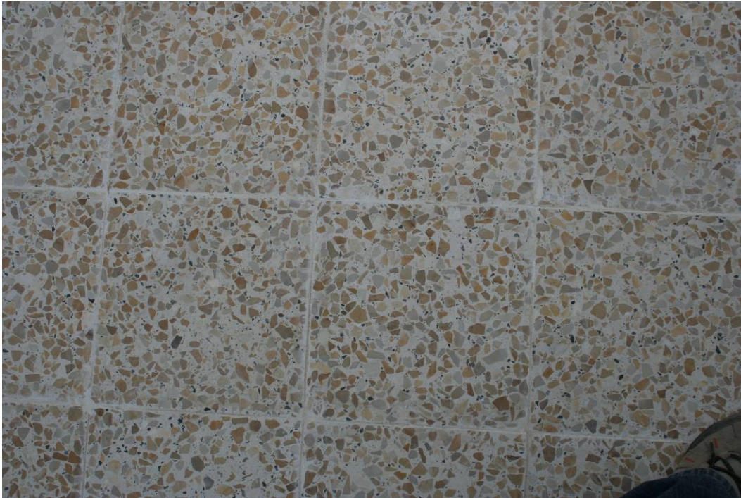
Site Photo 13. Terrazzo floor tile was used to finish most floors in the facility.
