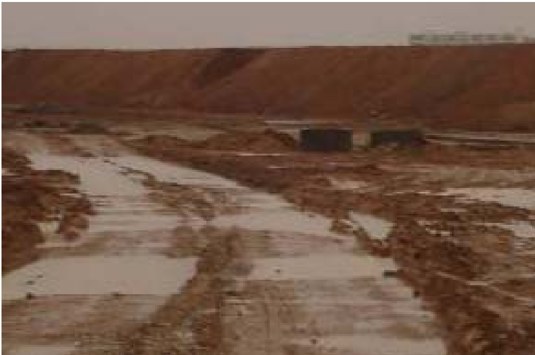
Site Photo 1. WST site conditions following overnight rain. (Photo from QA Report dated 3 Feb. 2006)
