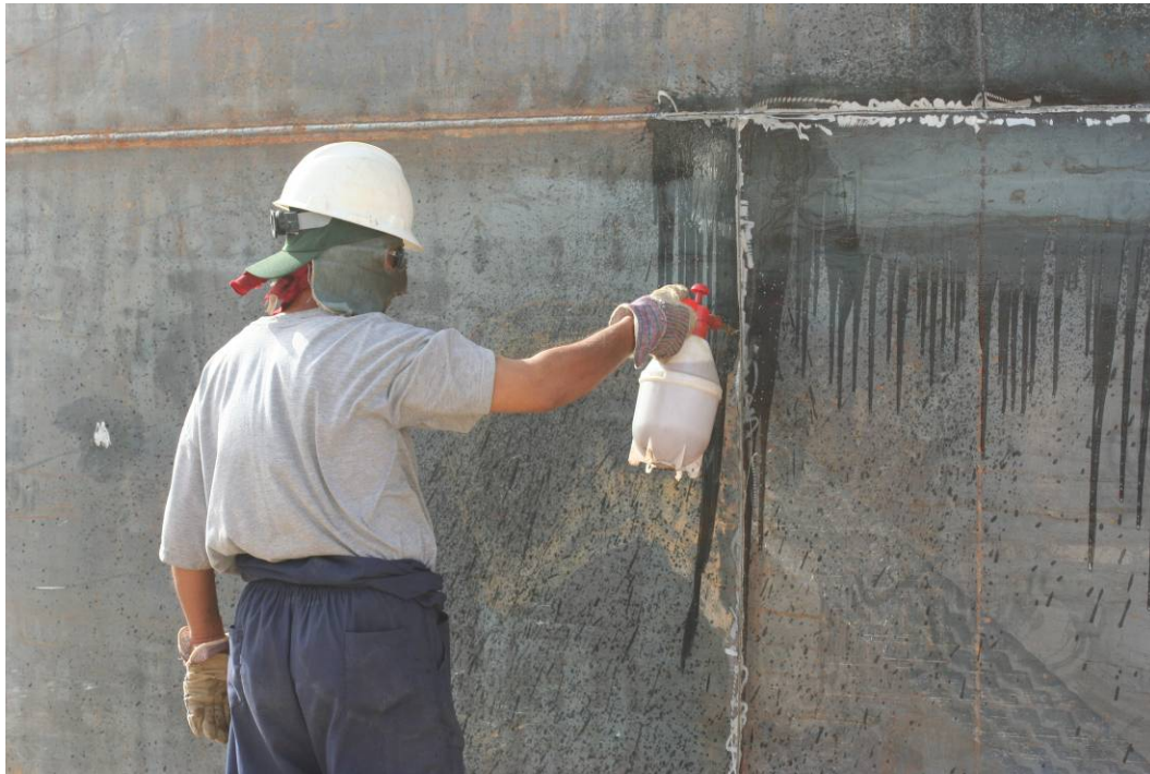
Site Photo 22. Diesel was sprayed on horizontal and vertical welds to conduct a penetrant test.
