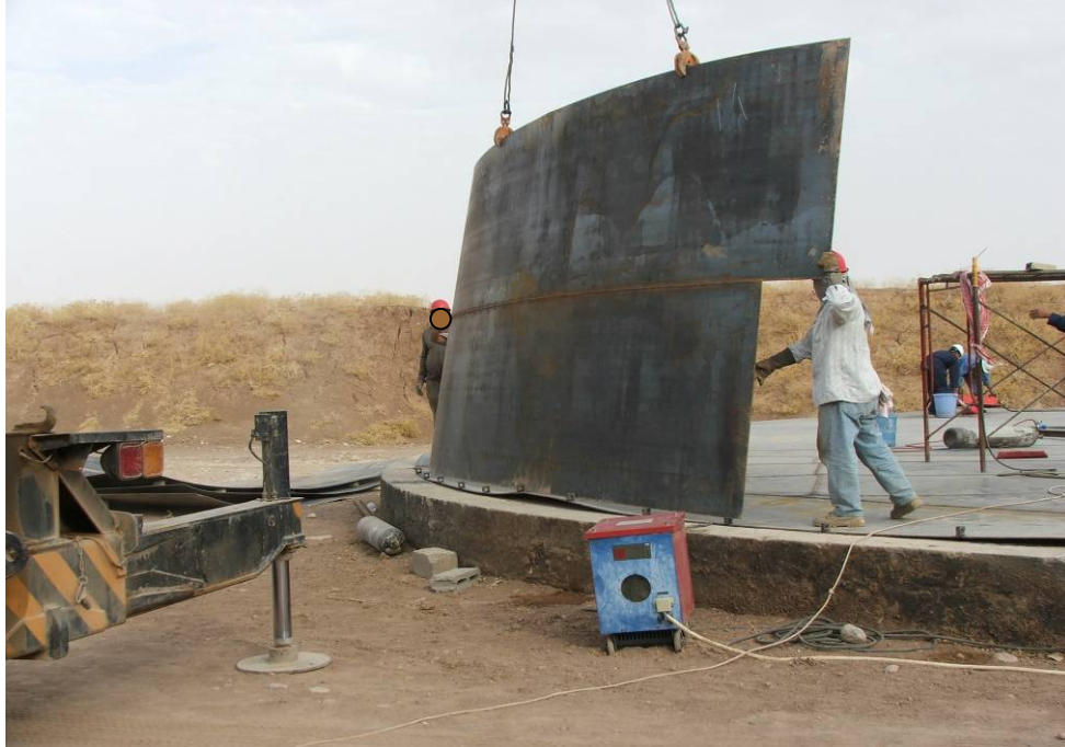
Site Photo 12. Steel plates were fabricated and placed on the base plates to form the tank's wall.
