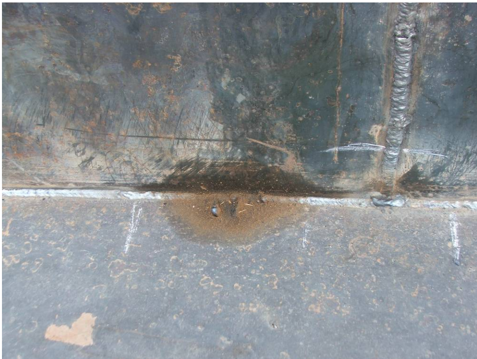
Site Photo 16. Diesel penetrated the welds within 24 hours of test.
