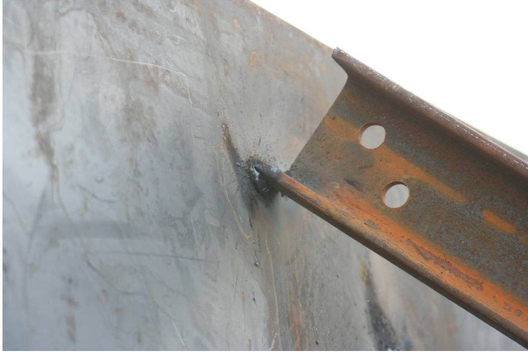
Site Photo 18. Top ends of steel beams are tack welded to the wall plates.
