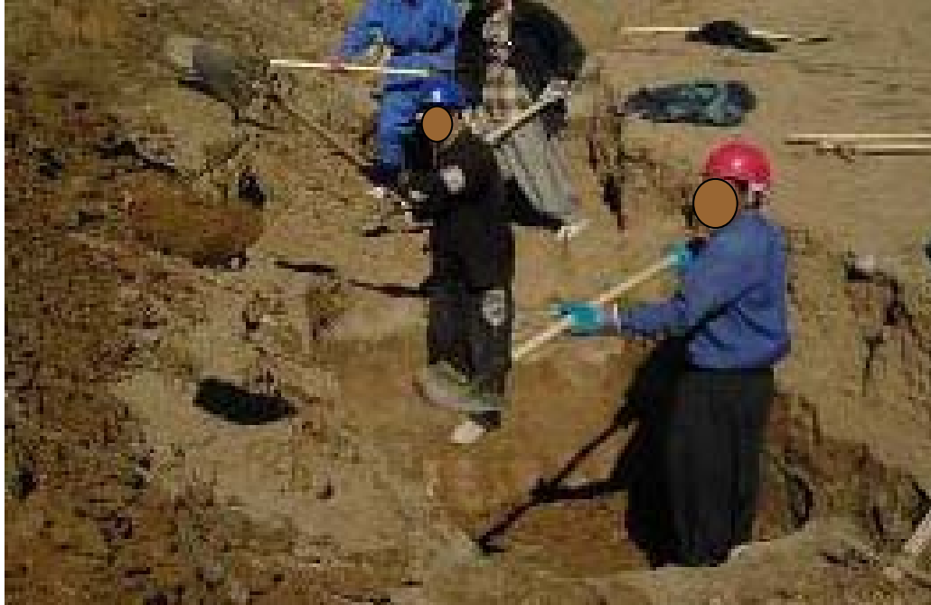
Site Photo 2. Workers have to re-dig footings after heavy rains. (Photo from QA Report dated 17 Mar 2006)
