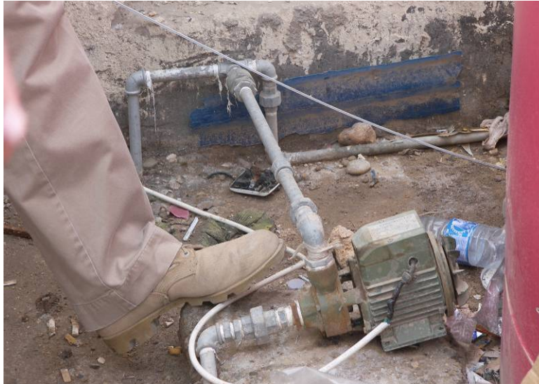
Site Photo 5. Water tank pump exposed to the outside elements
