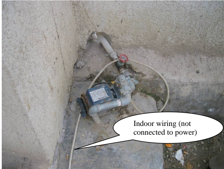
Site Photo 6. Exposed water pump connected to the main water supply line using indoor wiring. (Wiring is not connected to electrical power.)
