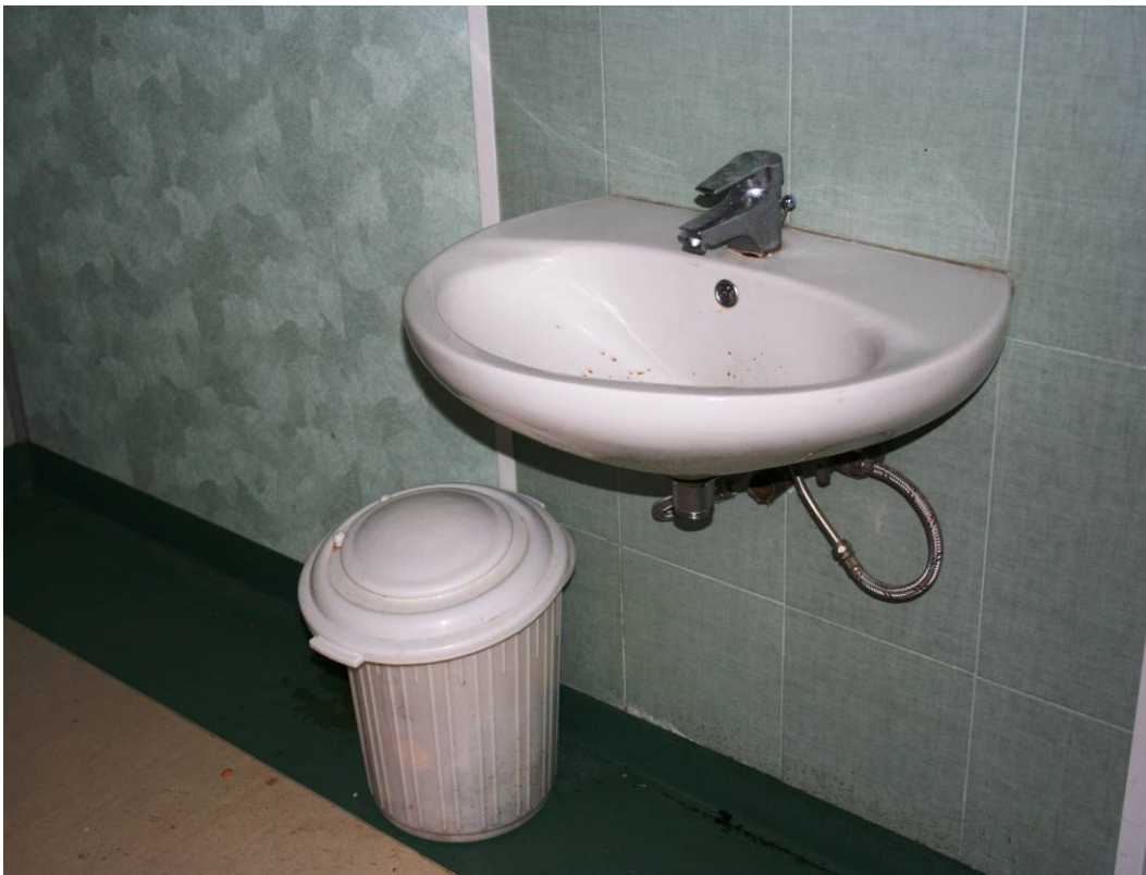
Site Photo 26. Drain pipe/trap was removed from patient care room sink.
