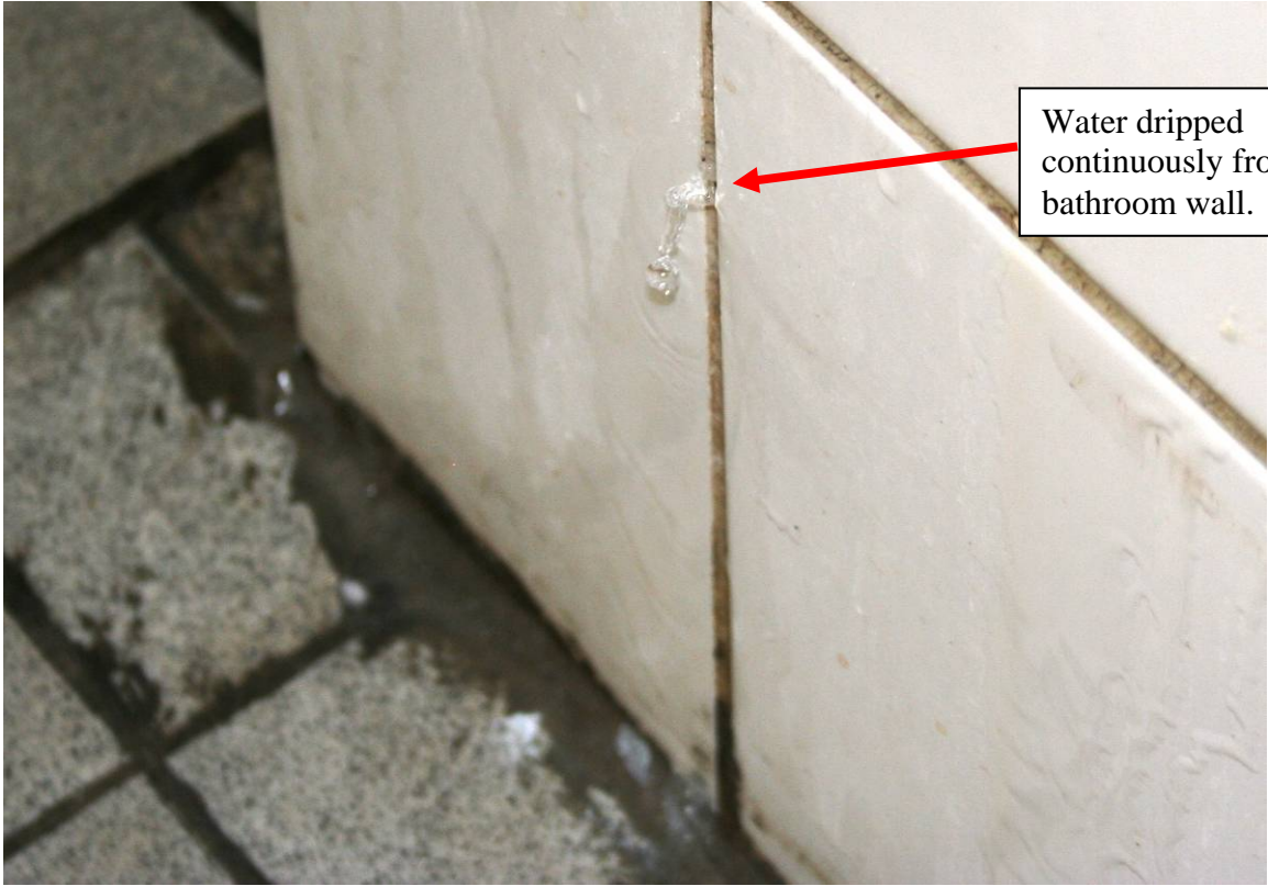
Site Photo 23. Steady dripping of water from a bathroom wall.
