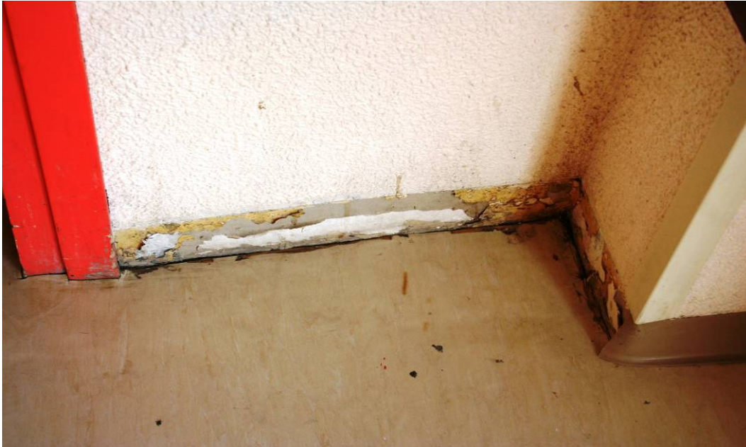
Site Photo 20. Water saturated and damaged wall.
