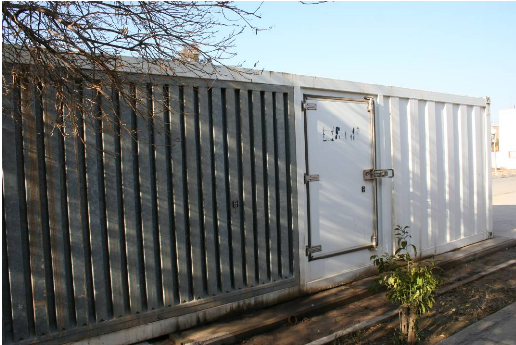
Site Photo 35. Generator installed pre-rehabilitation by World Health Organization.
