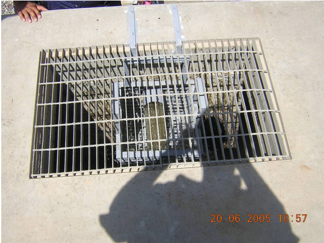
Site Photo 9. Inlet to septic tank was clean during commissioning. (USACE photo)
