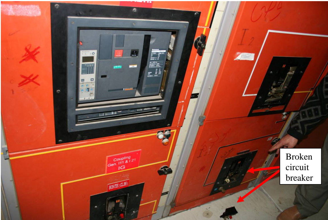
Site Photo 37. Broken circuit breaker that disabled switch gear equipment.
