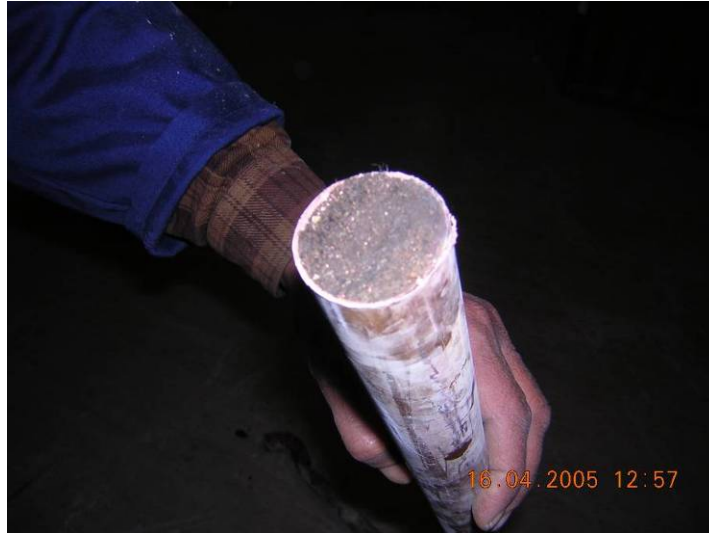
Site Photo 31. Plugged chiller water line before renovation. (USACE photo)
