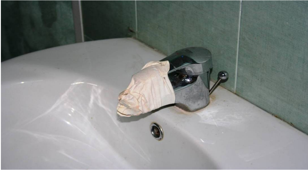
Site Photo 25. Some patient care room sinks were unusable.
