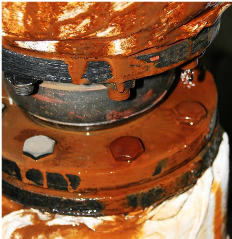
Site Photo 32. Evidence that rust contaminated water has leaked from a hot water line flange for an extended period of time.
