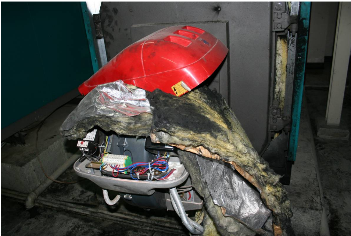
Site Photo 28. One of the three boilers was cannibalized for parts.
