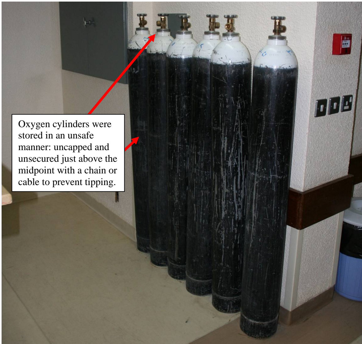
Site Photo 34. O2 bottles were stored in the hallway.
