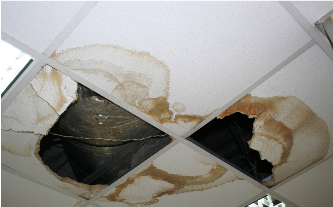
Site Photo 24. Damage from dripping water shown in Site Photo 23.
