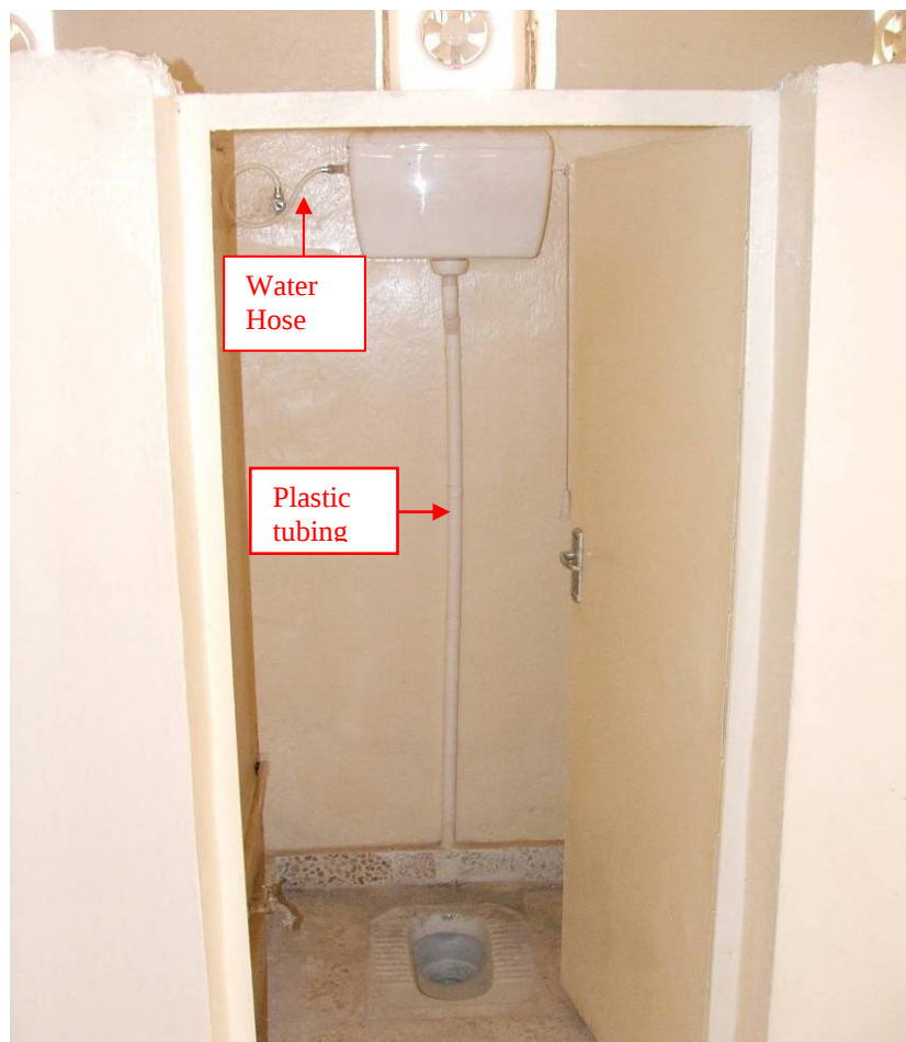
Site Photo 11. Water closet in ablution building
