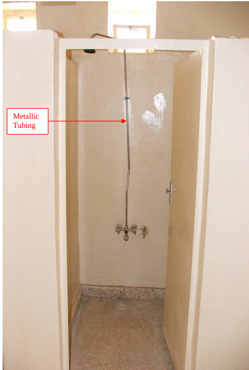
Site Photo 9. Shower in ablution buildings
