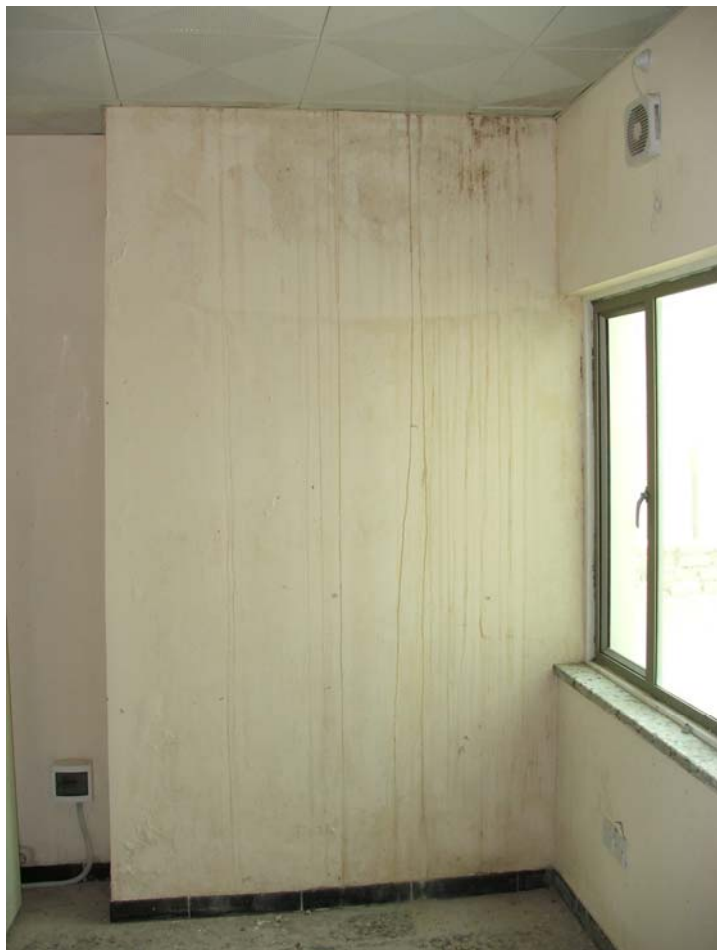
Site Photo 4. Water damage to wall
