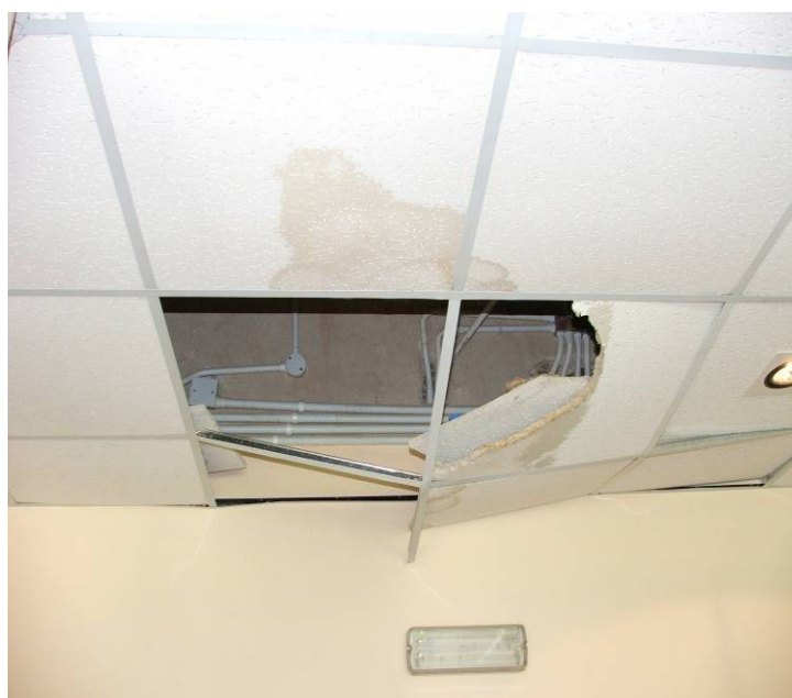
Site Photo 5. Water damage to ceiling
