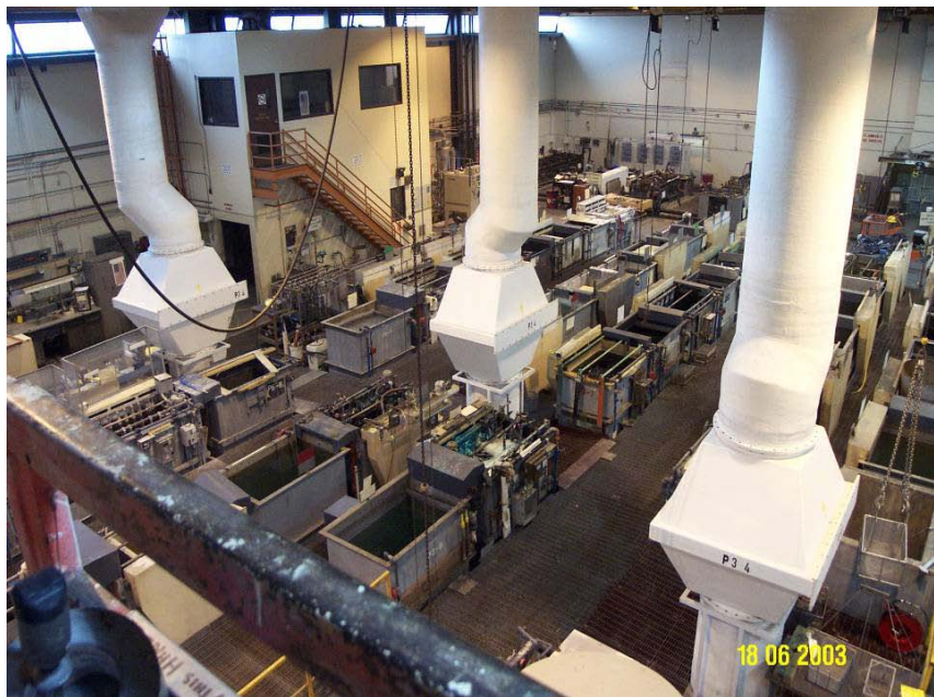
Figure 2-1. Chromium plating bath operation at NADEP.
