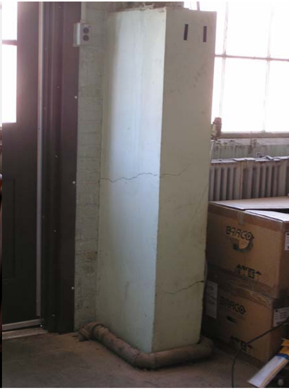
Figure 28: Pedestal 1 north: severely damaged pedestal.
