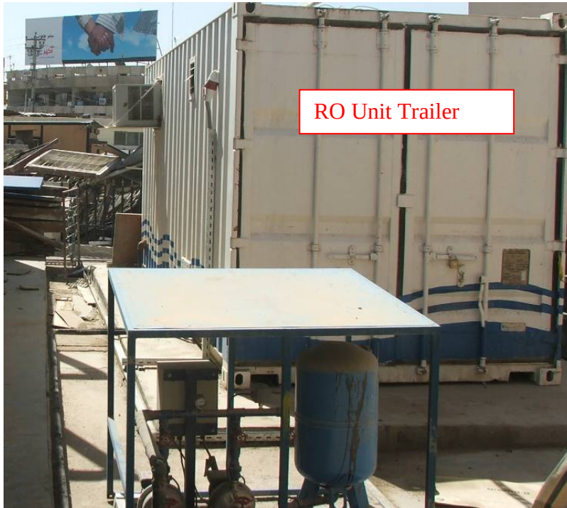
Site Photo10. Container housing the RO unit
