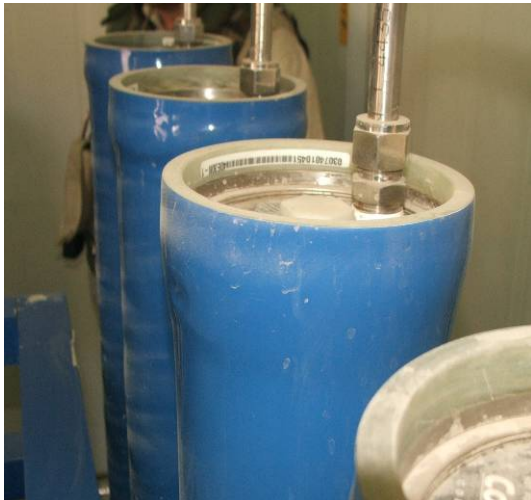
Site Photo 11. Pressure vessels containing RO membranes
