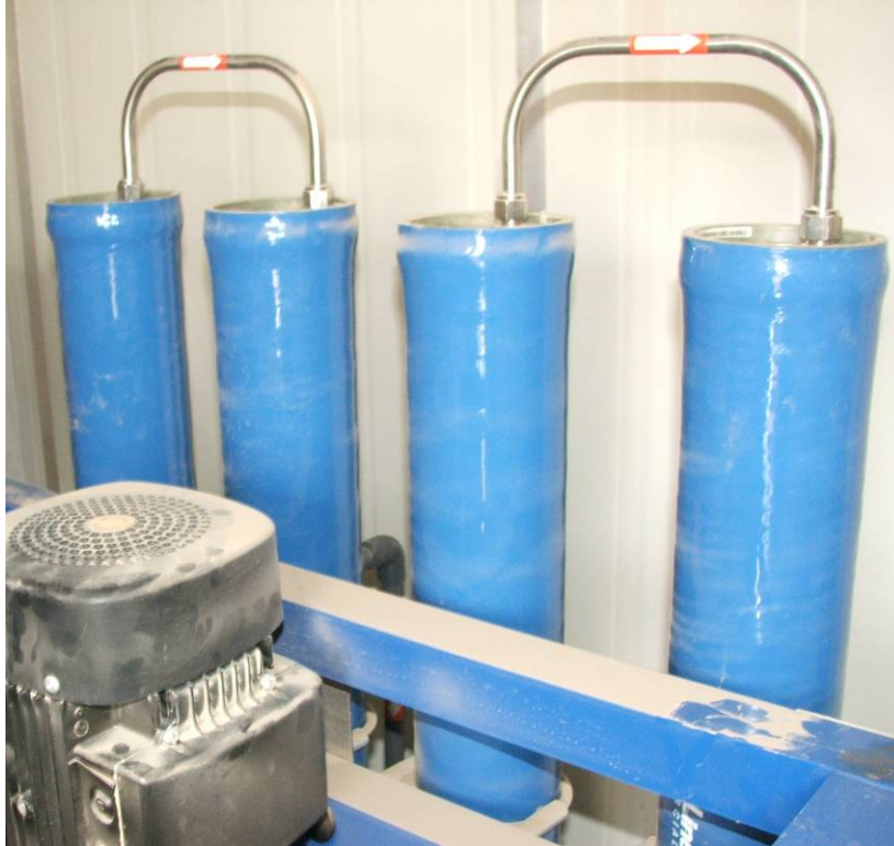
Site Photo 6. Pressure vessels containing RO membranes
