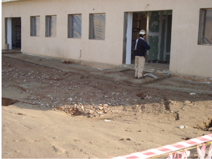
Photo 7: Lack of Grading that Contributed to Soil Settling at Kunduz ANA Garrison
