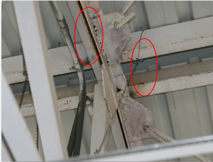
Photo 2: Rust on Steel Supports at Kunduz ANA Garrison
