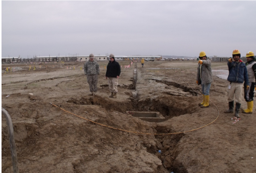
Photo 6: Roadbed Showing Settling at Kunduz ANA Garrison
