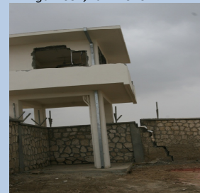
Photo: Guardhouse and wall on soil that has settled at Kunduz ANA garrison, Jan. 2010.
