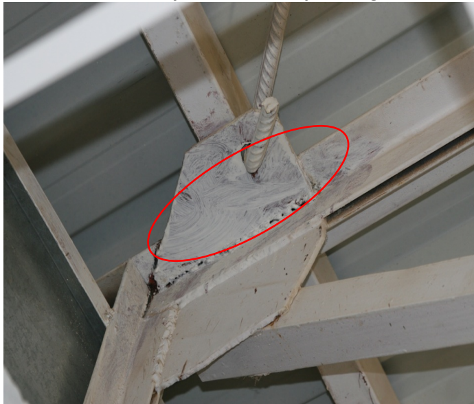
Photo 1: Poor Quality Welds on Sway Bracing at Kunduz ANA Garrison
