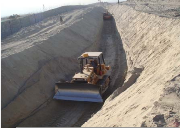
Photo 3: Anti-Vehicle and Flood Control Trench at the Gamberi ANA Garrison
