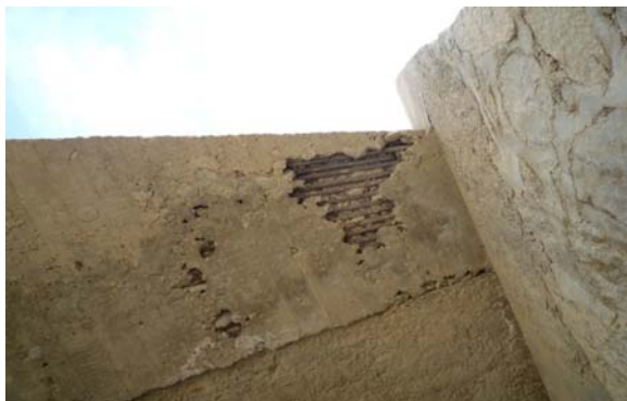
Photo 6: Exposed Reinforcement Bars on Underside of Culvert Deck over Drainage Ditch
