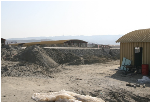
Photo 4: Grading at the Gamberi ANA Garrison that May Result in Poor Drainage
