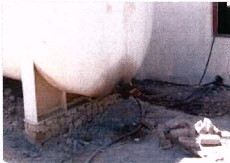
Photo 4: Power Plant 1 PRE-IMPROVEMENT —The 20,000 liter diesel fuel storage tank located at the outside rear wall of the main Power Plant 1 building. The tank is balanced on a platform of loose bricks with no spillage containment. Hoses are leaking fuel into the ground. The support deficiencies and lack of a spill containment area were documented requirements for the project in January 2008; however, no provision to improve this condition was made in the final scopes of work for the project. This photo documents the conditions observed by the SIGAR Inspection Team in May 2009. (Photo courtesy of Khowst PRT)
