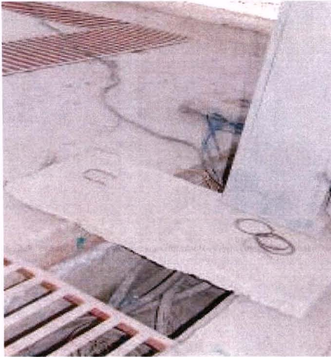
Photo 9: Power Plant 2 - View of the power distribution panel being balanced on one of two concrete slabs without any other means of support. (Photo—SIGAR)
