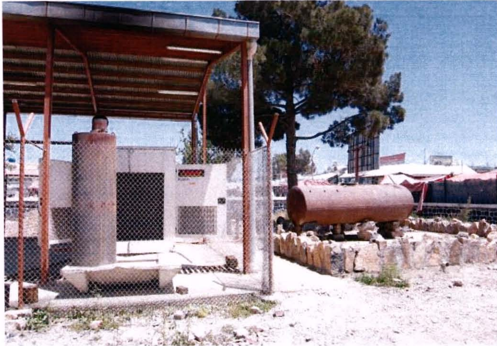
Photo 6: Power Plant 2. A view of the one of the 400kW generators relocated to an outdoor enclosure in the southern part of Khowst City at Power Plant 2. To the right is improvised diesel fuel storage tank, balanced on rocks and encircled by a containment area made up of large rocks cemented into place. Further the chain link fence surrounding the outdoor enclosure does not reach the roof and would not provide a barrier to anyone attempting to access the enclosure without permission. May 2009. (Photo—SIGAR)
