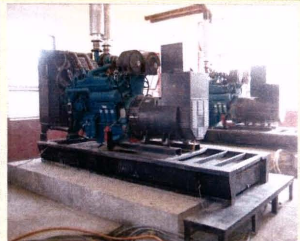
Photo: One of the three new generators installed at the Khowst City Power Plant 1 using CERP funds through a project initiated and overseen by the Khowst PRT: (Photo—SIGAR)
