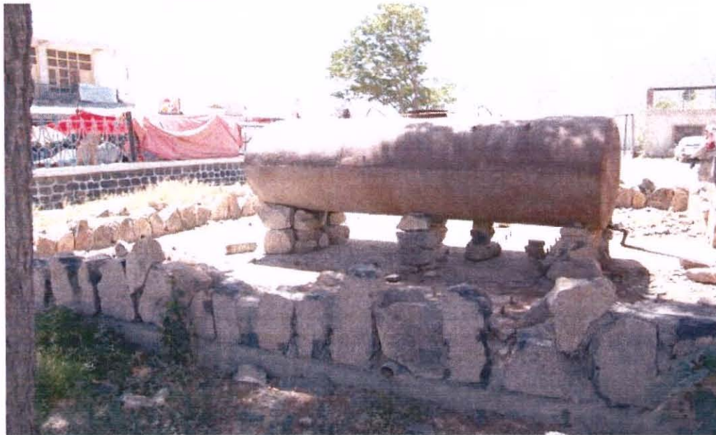
Photo 7: Power Plant 2. Corroded fuel tank used as a diesel fuel reservoir. The tank is supported by loose rocks and the spill containment wall is inadequate (Photo—SIGAR)
