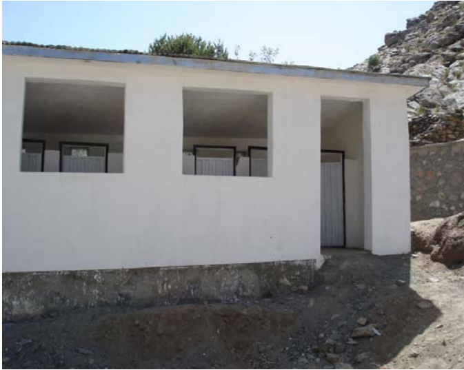
Site photo 2: View of the latrine containing inadequate opening sizes for refuse removal. (Photo provided by SIGAR)
