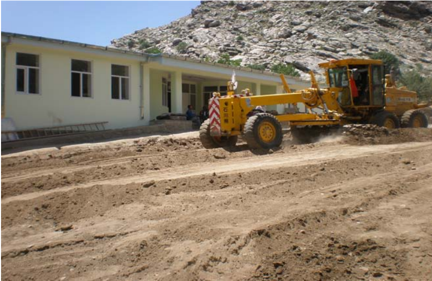
Site Photo 6: View of grader attempting to level the ground in front of the school house in mid- July. This grading improved, but did not solve, the ground erosion problem because there was no follow-up compaction of the soil. (Photo provided by Kapisa PRT)
