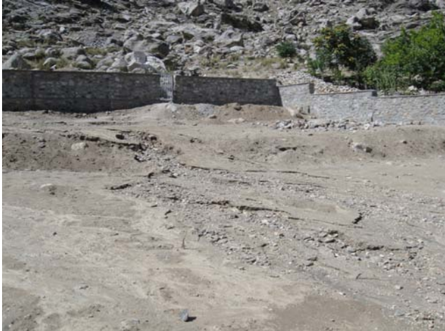
Site Photo 8: View of 2 meter high stone masonry perimeter wall at the rear of the school compound. The significant level of erosion can be seen. The perimeter wall parallel to the slope can be seen on the right. (Photo provided by SIGAR)
