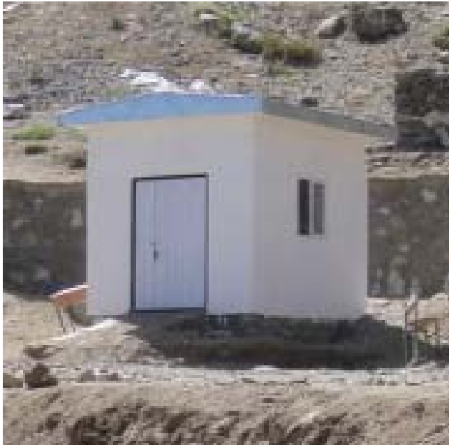
Site Photo 3: View of generator house which lacks proper exhaust venting as required in the statement of work. (Photo provided by SIGAR)
