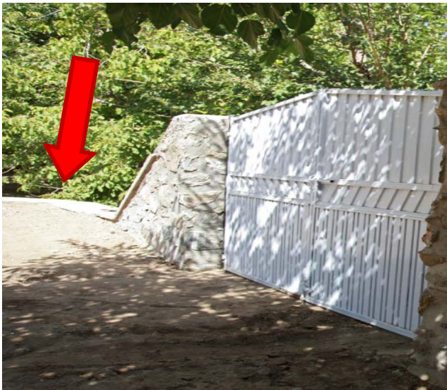
Site Photo 9: The top of the 2 meter perimeter wall can be seen (indicated by red arrow). During the site grading, soil was placed against the perimeter wall, bringing the grade elevation up to the top of the wall in some areas. (Photo provided by SIGAR)
