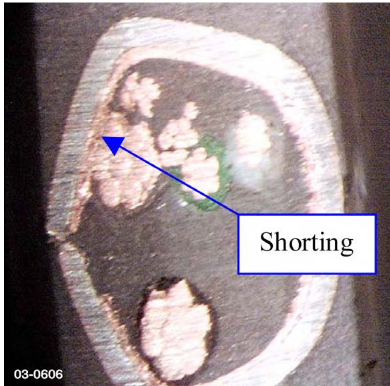
Figure 87. Shorting between power wire and metal housing
