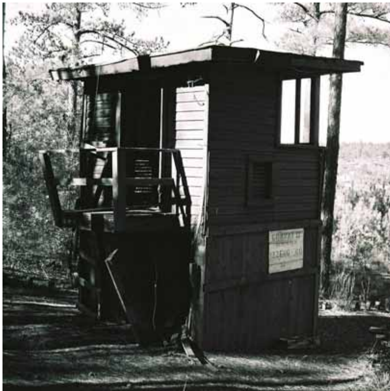
Figure 513. Remnants of 1950's observation tower on Combat II Range, Fort Jackson, SC, June 2004.
