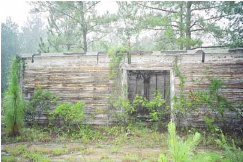
Figure 528. Remains of WWII Range Target Shed Bldg R161, Fort Gordon, GA, January 2004.
