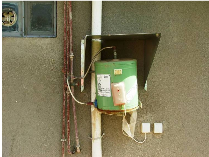
Site Photo 15. Water heater outside administration building
