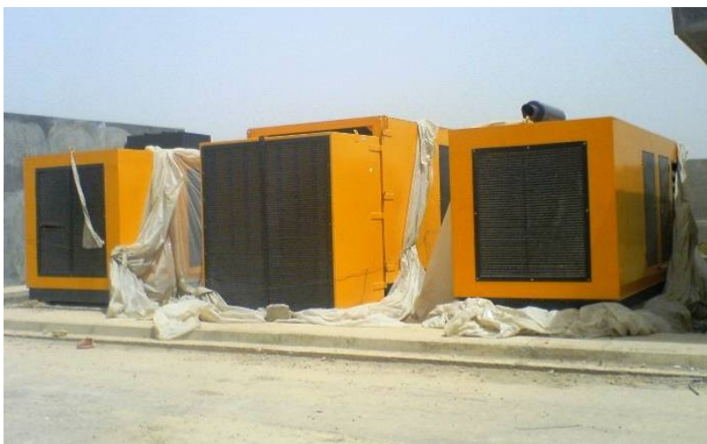
Site Photo 13. Generators for the courthouse (2) and the annex (1) (Photo provided by USACE)
