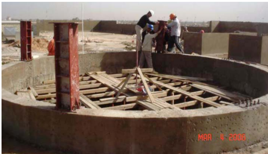
Site Photo 9. H-Columns anchored to dome concrete base (Photo provided by USACE)
