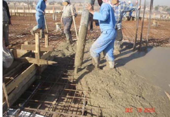
Site Photo 3. Concrete placement for roof slab pour (Photo provided by USACE)
