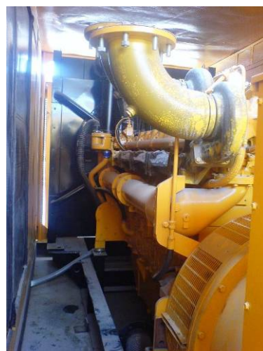
Site Photo 14. Interior of the generator enclosure (Photo provided by USACE)
