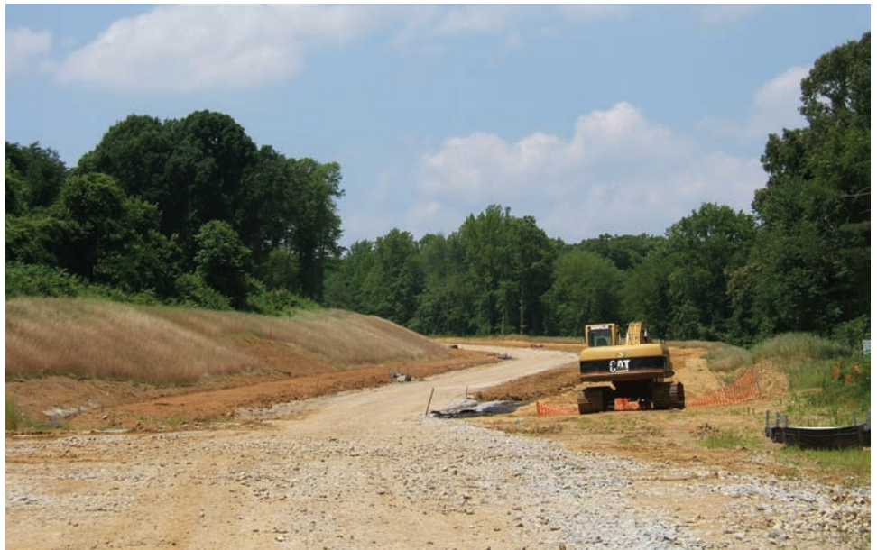
Figure 4: Construction of a New DAR Road at Fort Belvoir (Main Post) in Fairfax County, Virginia
