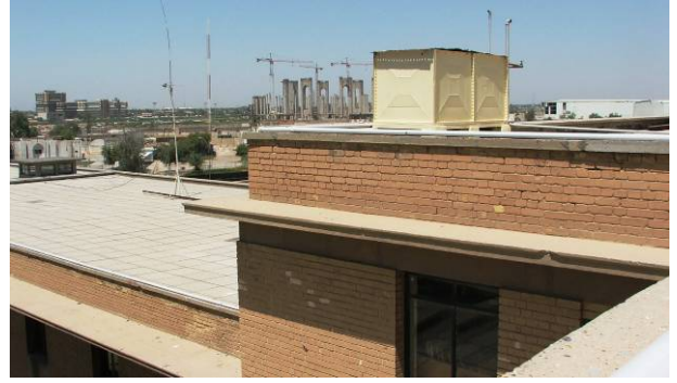
Site Photo 17. Roof top galvanized water tank
