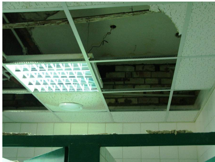
Site Photo 22. Water damage to the suspended ceiling
