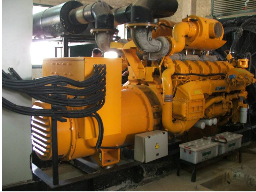
Site Photo 25. One of two Perkins 1,250 KVA generators
