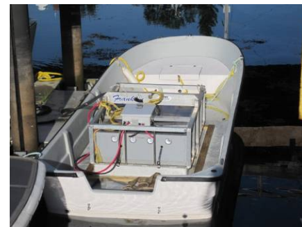
Figure 5: 20' Launch Containing Battery Bank
