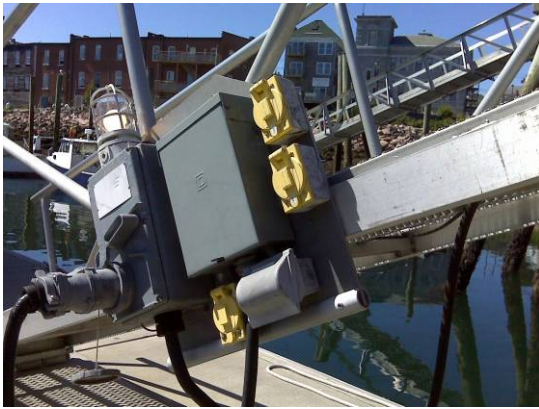
Figure 7: USCG Pier Electrical Panel and Connection
