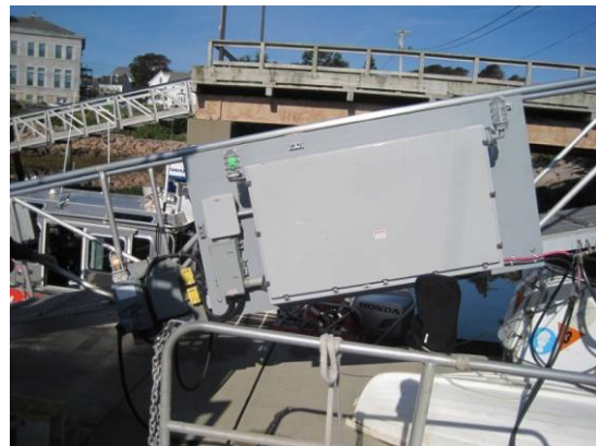
Figure 8: USCG Pier Electrical Panel and Indicator Lights
