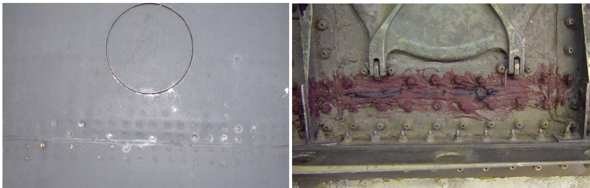
Figure 27-38: A Visual Inspection of the Exterior Surface Indicated Corrosion Pillowing (left) While the Interior Showed Sealant Added (red) Indicating Maintenance for Same (right).
