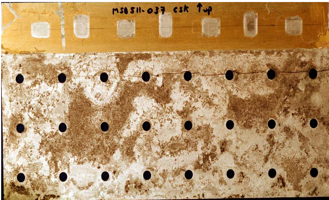
Figure 16-3: Faying Surface of the Countersunk Sheet of Specimen #037 Before and After the Removal of Corrosion Products.
