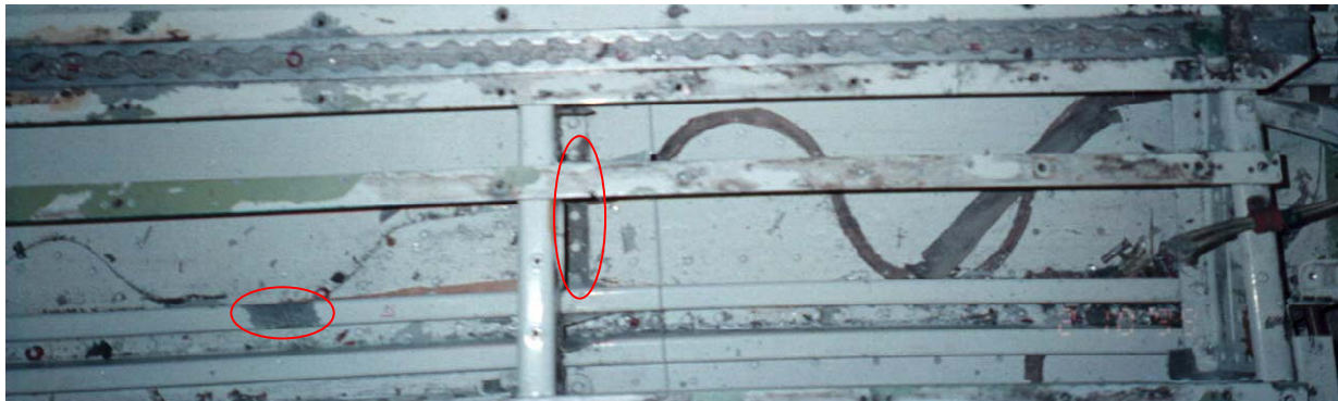
(a) White paint over primer (corrosion circled).
