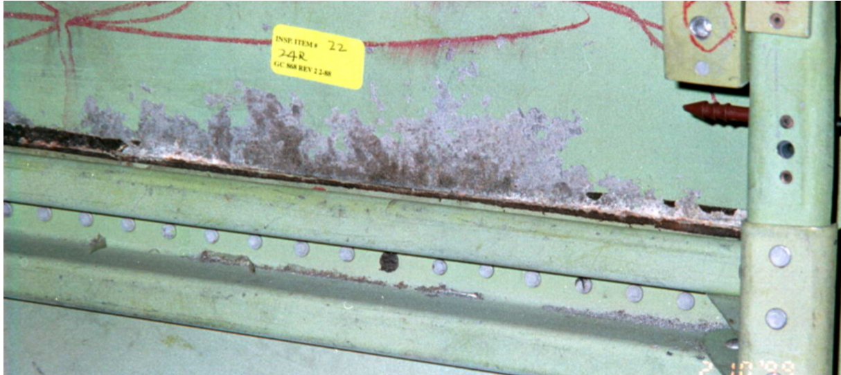
Figure 27-16: View of Surface Corrosion on INBD Side of Upper Skin at Lap Joint.
