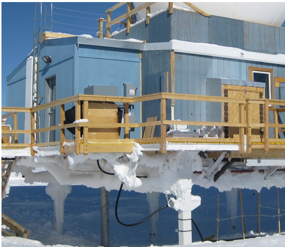
Figure 24. View 12 showing location (inset), thermal, and visual image of the of the southwest corner where the west vestibule connects to the main building
