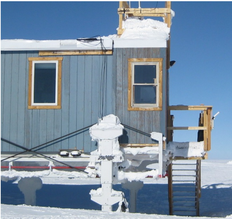
Figure 19. View 7 showing location (inset), thermal, and visual image of the eastern end of the South exterior wall in the vicinity of the main room and east vestibule.
