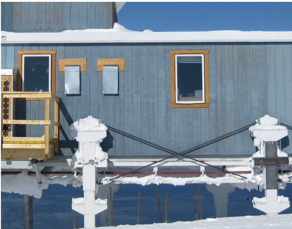
Figure 21. View 10 showing location (inset), thermal, and visual image of the south exterior wall in the vicinity of the kitchen.
