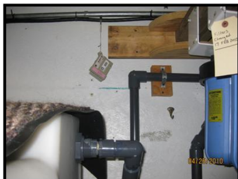
c. Mechanical Room
