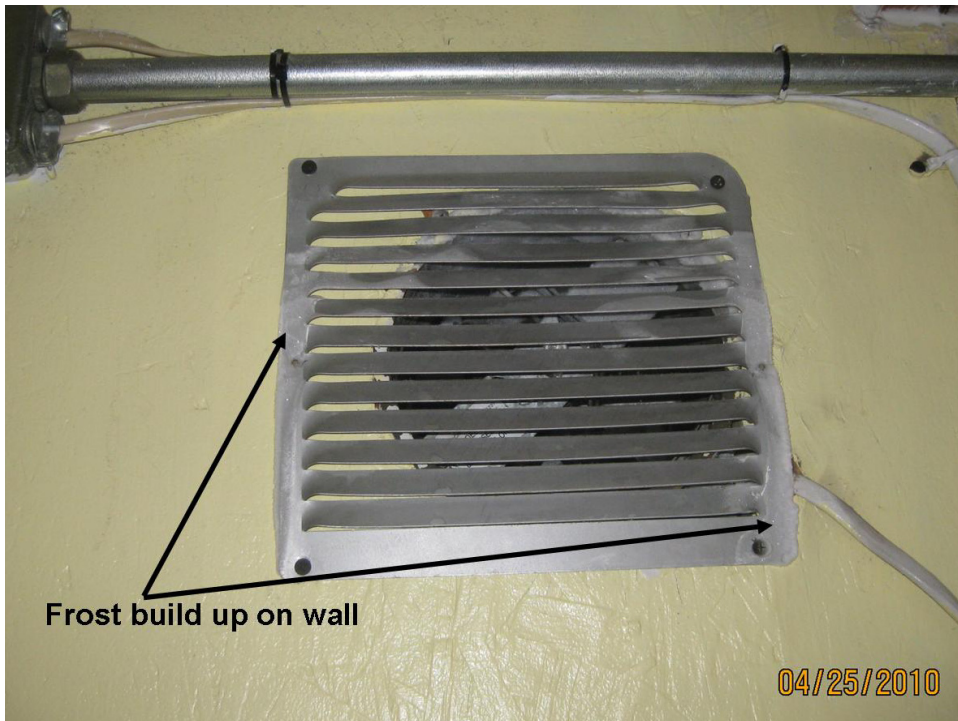
Figure 41. IR image of both the clothes dryer and through-wall vent in the laundry room/bathroom. The visual image is a closeup of the through-wall vent noting frost buildup from cold air infiltration.
