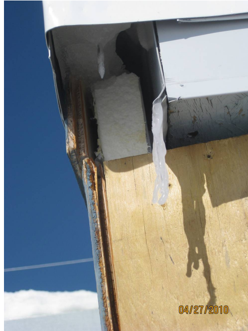
Figure 25. Closeup of the southwestern corner of the original main building showing the gap between the materials of the original exterior and the recent re-sheathing.
