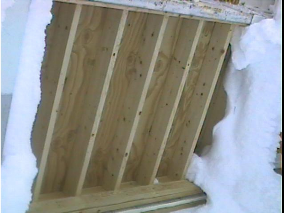
Figure 29. View showing thermal and visual image of heat loss through base of unheated eastern vestibule.
