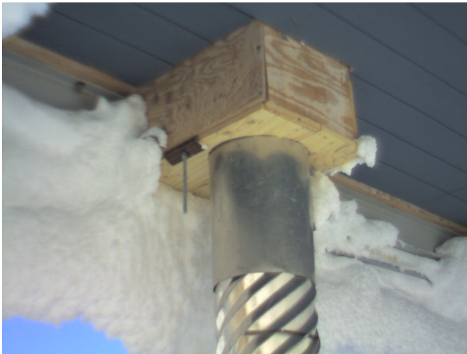
Figure 31. Base of the building, IR and visual images of the sewer outfall pipe.
