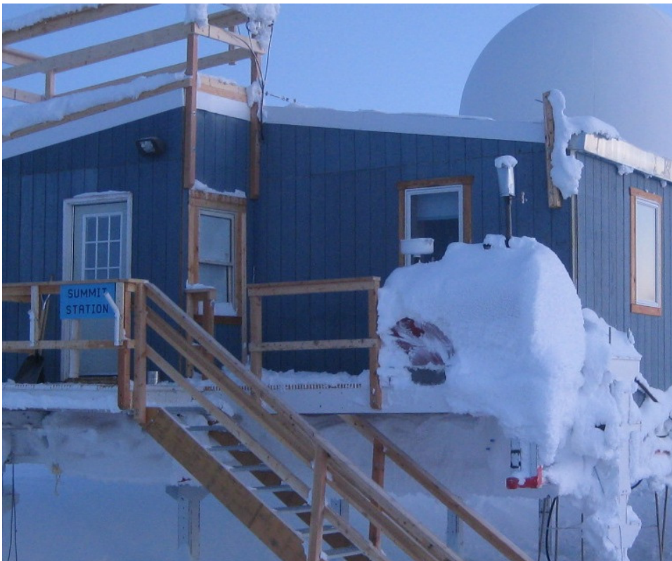
Figure 17. View 4 showing location (inset), thermal, and visual image of the northeastern corner including the office and eastern unheated vestibule.
