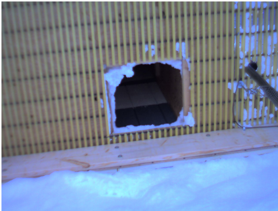
Figure 32. Base of the building, IR and visual images of the kitchen air intake vent.
