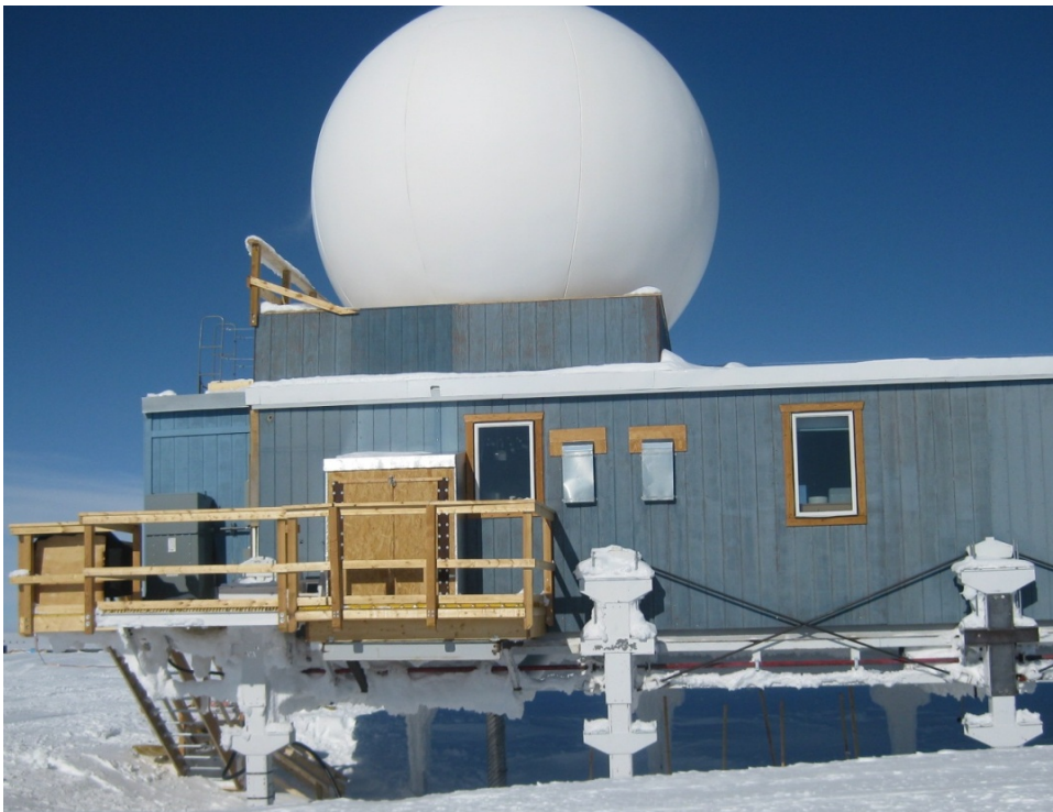
Figure 23. View 11 showing location (inset), thermal, and visual image of the of the south exterior wall west end in the vicinity of the kitchen.
