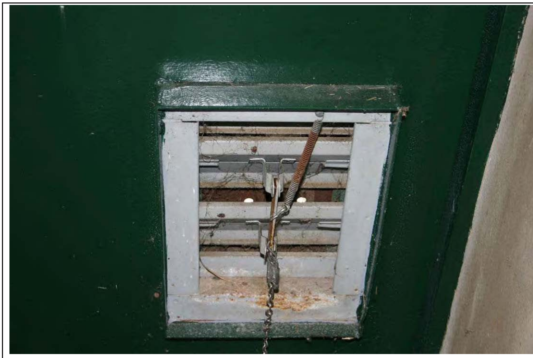
Figure E-28. Door air vent.
