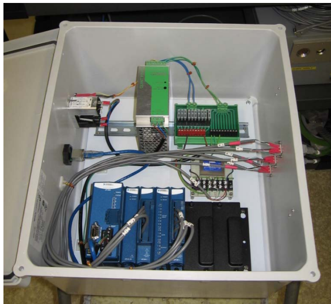
Figure 7-2 – Interior View of SBVS Fieldpoint Unit
